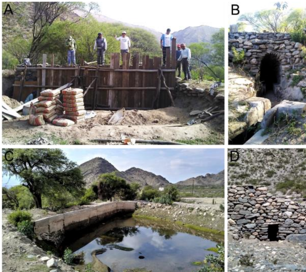
Figure 9.22: Community-led projects in the Indian Community of Quilmes. a) Structural renovation to reinforce the stone dam of Talapazo with a concrete wall to return the infrastructure to community service after several years of neglect; b) The back of the dam in Talapazo with attached the beginning of the stone channel leading to lower farm plots; c) The reconstructed dam halfway the villages of Quilmes Centro and Rincón de Quilmes. d) The ruins of the ancient dam in the archaeological site of Quilmes. October – November 2018.
