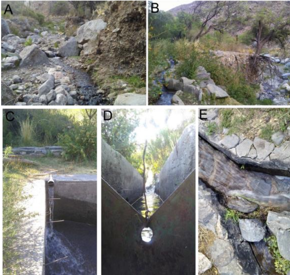
Figure 9.21: a) The upper stream of the seasonal river of Talapazo at the start of the ditch that conveys the spring water into the stone canalisation built through the national subsidy in the 1990s; b) The ditch continues along the dry riverbed, threatened by the erosion caused by the amount of water brought by the growing of the river; c) In proximity of the first houses of the village, the water coming from the stone canalisation can be directed into a cistern, depending on the turn of each family, and from there it passes through a desander filters before flowing into the pipeline; d) To regulate the flow into the stone channel or the hoses according to the cyclical shifts, a metal plate is either lifted or put down in order to fill the contiguous cistern; e) The water flowing down the principal stone canalisation and detail of the opening of a ditch that enables directing water to an household plot. October 2018.
