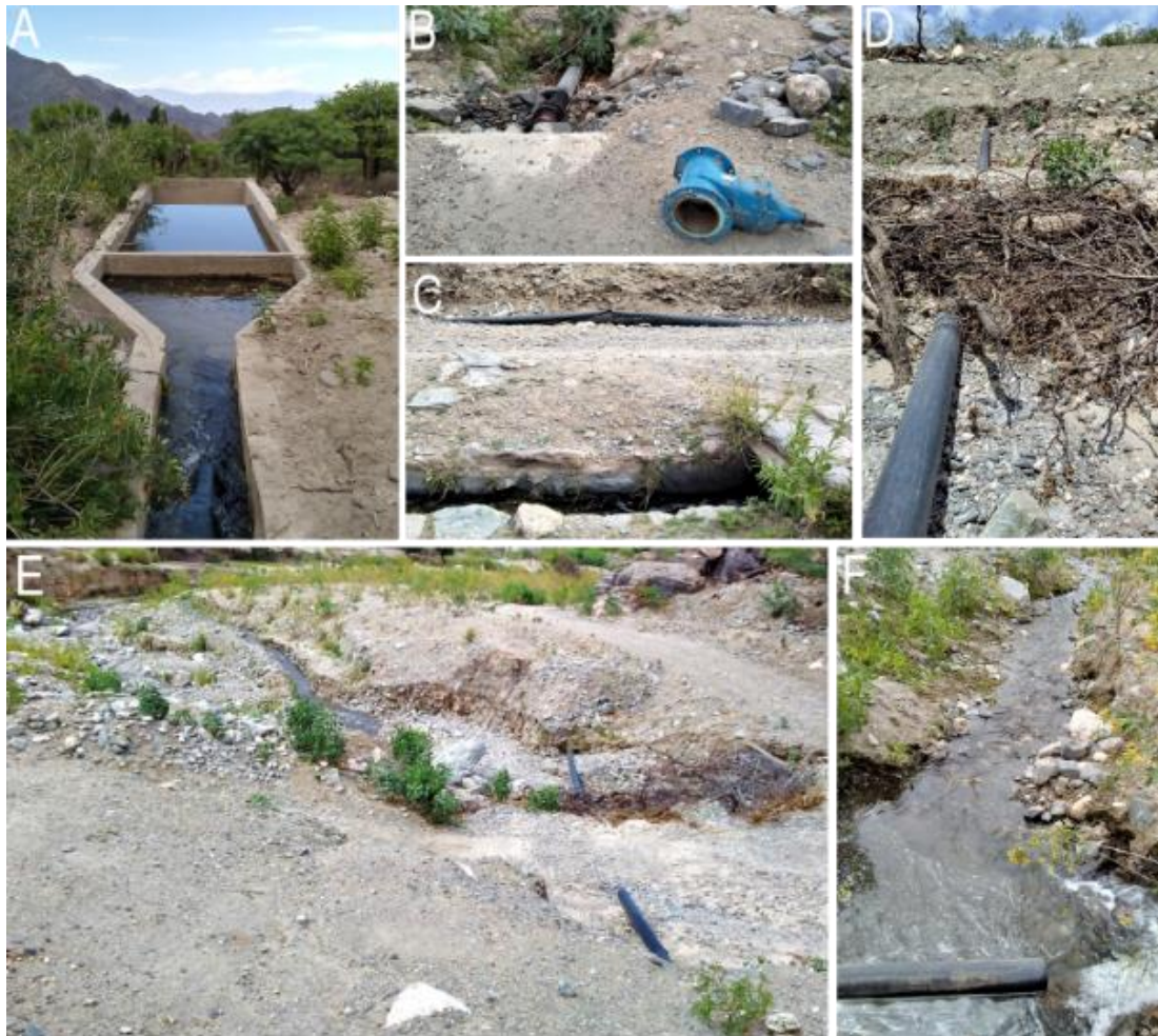
Figure 9.23: a) The first desander at the beginning of the WB-DCI water pipeline system in Rincón de Quilmes; b) An element of the system departed from a pressure load breaker; c) In the background, the remain of a hose went off because of excessive water pressure, and the pre-existing stone ditch where the water has returned to flow; d) The main system tube buried under a mudslide; e) The dry riverbed from the top of the compacted mudslide with the abandoned tube and the ditch that was dug for the emergency; f) Detail of the beginning of the emergency ditch. November 2018.
