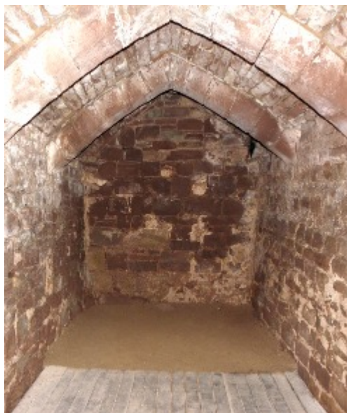
Fig. 11. Goodrich Castle. Interior of the late C13 or C14 prison cell with the lower courses of the keep wall to the right.
