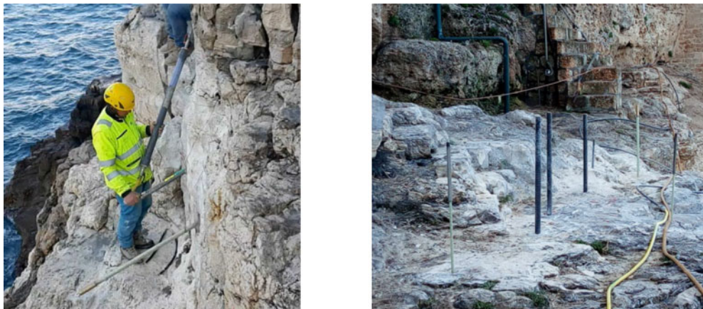
Figure 9. a) Technician during injection MasterEmaco A 60 in CB1/2; b) anchor in FT2 zone 1.
