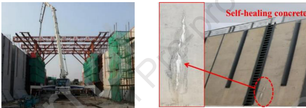
Fig. 10. (left) Pouring of the BBSHC during the reconstruction of the Mangdao River ship lock chamber in China; (right) crack healing (after four months) in the channel walls of the ship lock [93].
