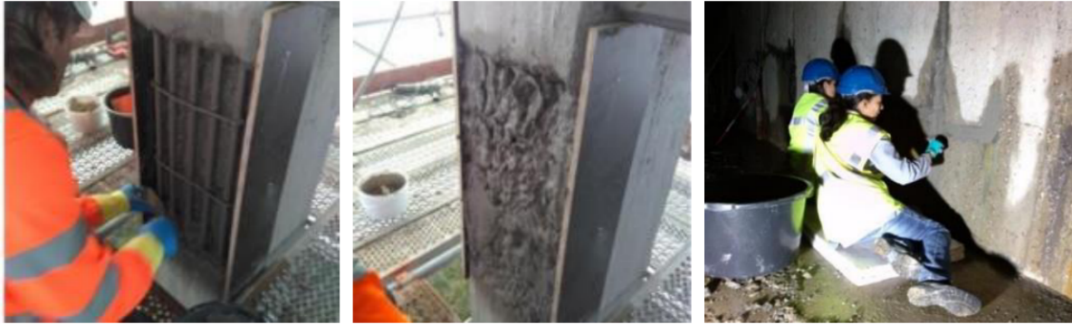
Fig. 11. Use of bacteria-based self-healing mortar (BBRM) for: ( left and middle ) on-site structural repair of damaged steel-reinforced concrete; and ( right ) manual repair of actively leaking cracked concrete basement walls [20].
