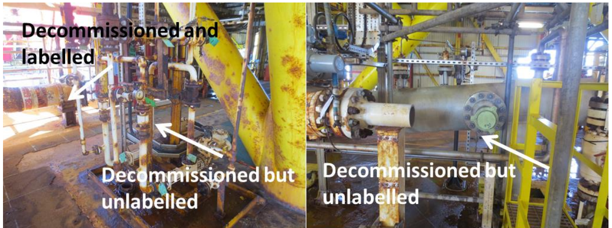
Figure 7-11: Poor identification of decommissioned equipment. Source: Author
