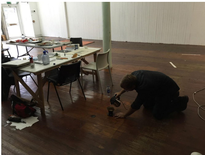
Fig. 45. Andy imagines the hole in the floor.
