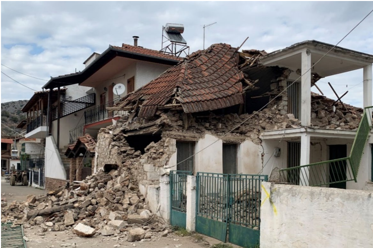
Fig. 15 Out of plane collapse due to poor connection between the roof and the underlying masonry and no rigid top floor, Damasi, Greece
