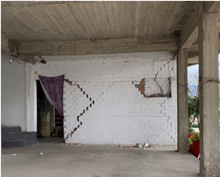
Fig. 9 In plane shear failure of poorly confined masonry wall due to door opening in Mesochori
