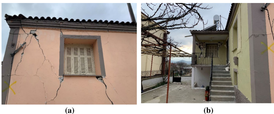
Fig. 19 Shear cracks due to diagonal tension in domestic masonry buildings in Mesochori
