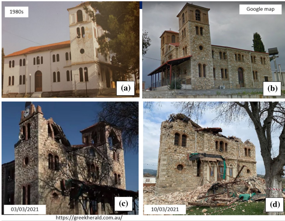
Fig. 26 Church of Agios Dimitrios at Mesochori a view from the 1980s; b before the earthquake; c after the main event of 3/3/21; d after the aftershocks on 10/03/21
