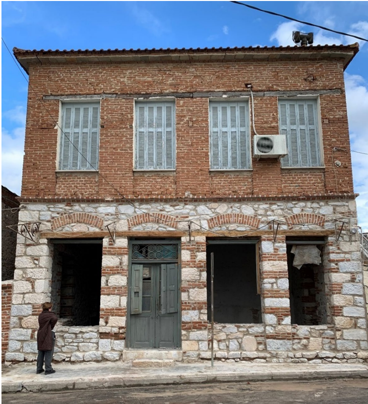
Fig. 12 Masonry house with large openings and wooden lintels above openings in Tyrnavos. The ground floor is made of stone masonry while the first floor is made of clay bricks
