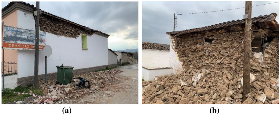
Fig. 18 Delamination of a the upper part; and b entire wall of a masonry buildings in Mesochori
