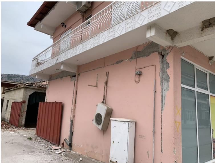
Fig. 8 Damage of infill walls in a RC building due to out of plane bending and shear damage in the column due to in plane infill behaviour in Damasi
