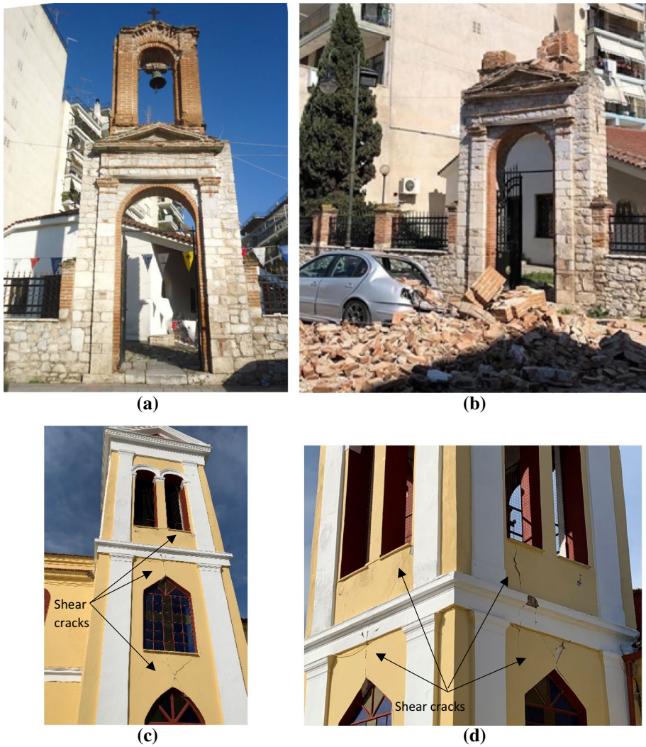
Fig. 25 a Bell tower of church of Agios Ioannis in Tynavos before the 3/3/2021 event (source: Tirnavospress.gr); b out of plane failure after the earthquake; c and d shear diagonal cracks between openings at the bell tower of the church of Agia Paraskevi in Tynavos
