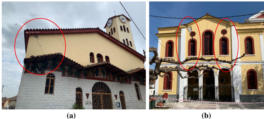
Fig. 28 Damages (within the red ellipses) in the corner and perimeter wall of churches at a Damasi (church of Agios Nikolaos); and b Tyrnavos (church of Agia Paraskevi)
