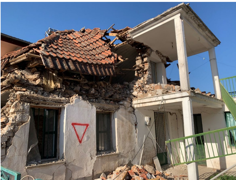
Fig. 16 Pounding failure due to different dynamic characteristics of structural components
