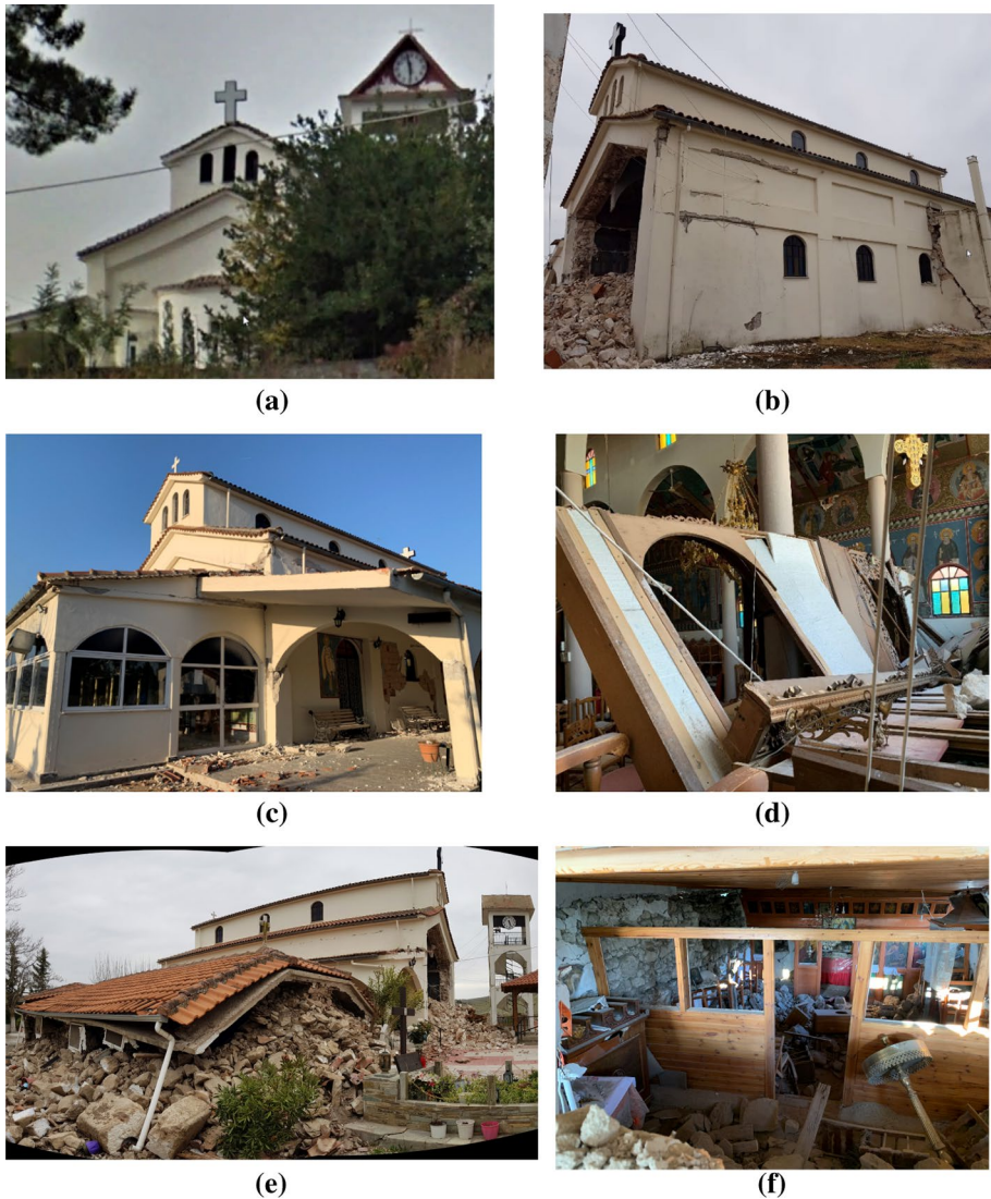
Fig. 29 Church of Agios Nikolaos at Koutchochero: a before the earthquake (picture taken from Google maps-street view), b North side of the church after the earthquake of March 2021; c west side of the church; d non-structural damages inside the church; e older, Agios Nikolaos chapel; f interior of the chapel of Agios Nikolaos
