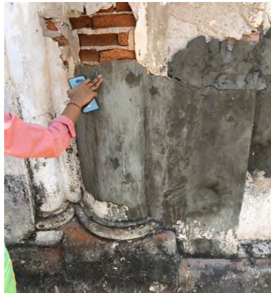
Image of unsuitable concrete render repairs on the south gable wall of Dipinkara Shrine
