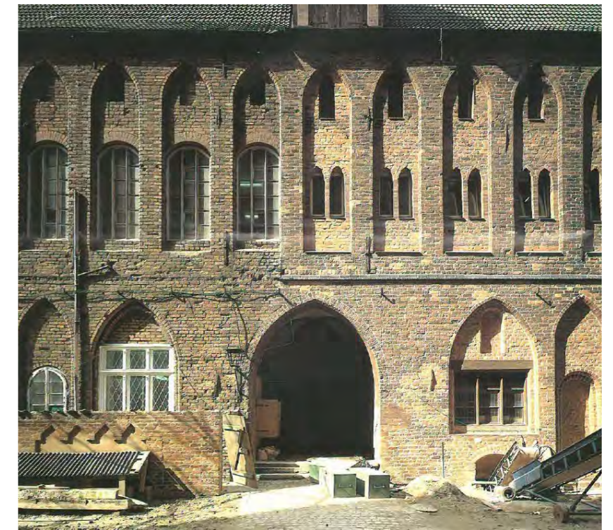
On the ground floor of the restored facade (right), pre-reunification work had replaced carved baroque or earlier mullion-and-transom windows with speculative reconstructions. The facade on the left retains its building biography, and was repairable.
