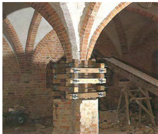
Pre-reunification column and vault repairs in the Ratskeller used hard new brick and cement rendering (rear of the image). The repairs under Purcell's direction conserved brick ribs and lime-washed the vaults are in the foreground. The 1890's brick casing to the column was repointed and limewashed too.
