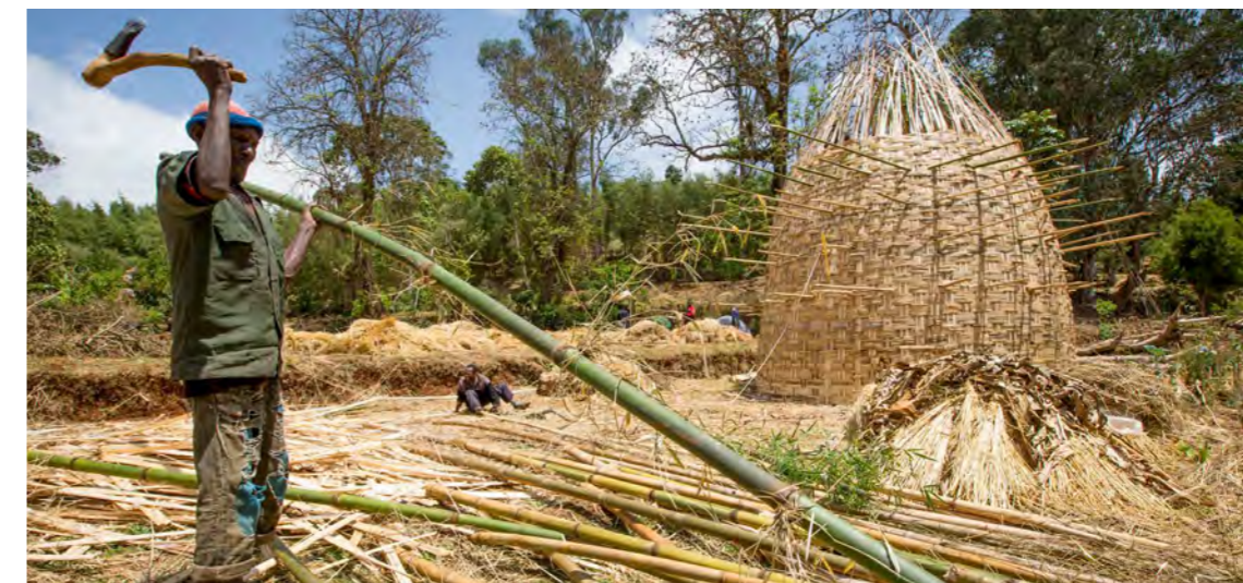
Figure 7 – The skills are as important as the building – Dorze Woven Bamboo House, Ethiopia
