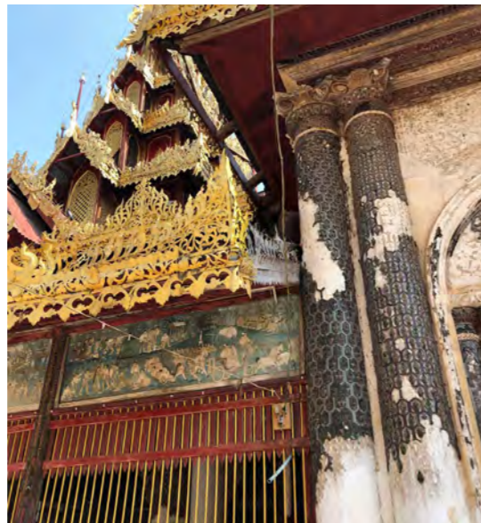
Junction on the north facade of the Hna-Kyeik-Shit-Su Shrine showing the loss of external finishes on the relief columns
