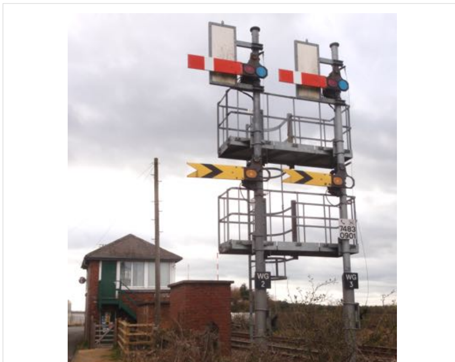
Figure A.144b: Winning Signal Box retains this noteworthy semaphore signal installation on modern posts. (Author 2019)
