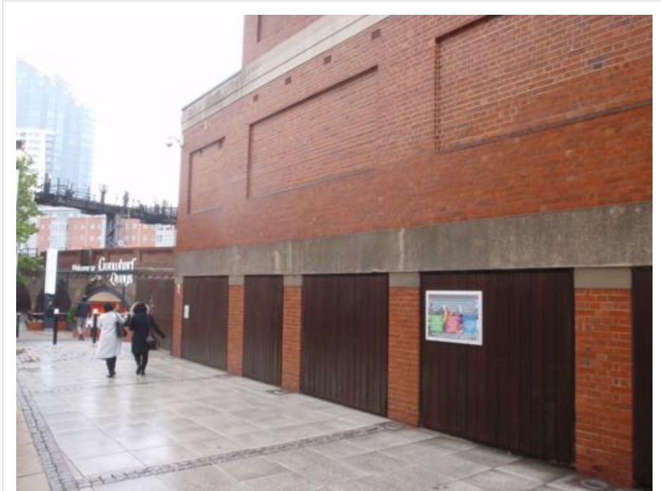
Figure A.100b: Street level view of Portsmouth Harbour Signal Box, showing voids with potential for retail use. (Author 2016)
