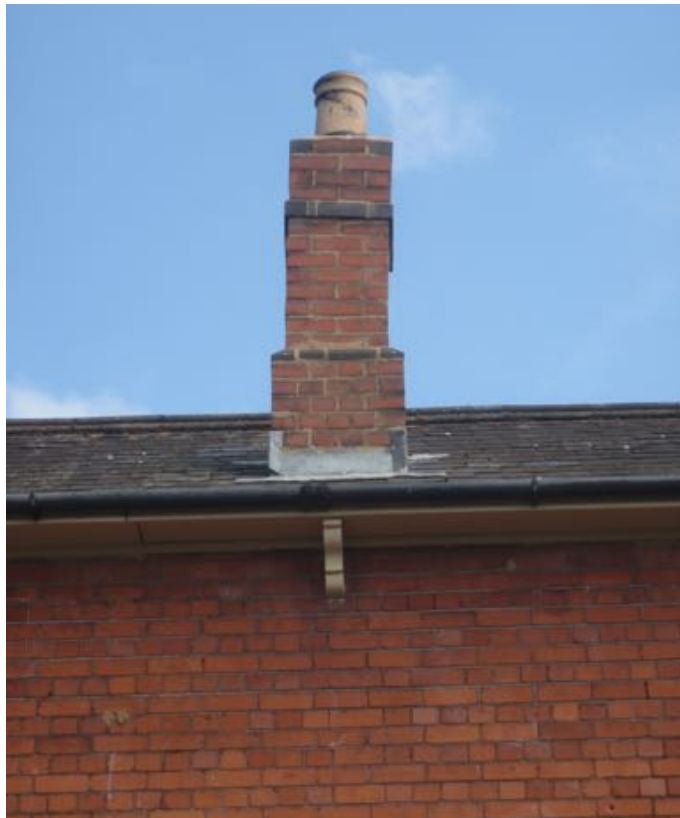
Figure A.101e: Chimney rebuilt with pre-existing lean for authenticity, Princes Risborough North Signal Box. (Author 2018)
