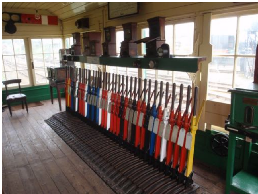
Figure 6.3: Operating floor of Chappel & Wakes Colne Signal Box. Visible on the equipment shelf are some explanatory display labels. The closest railway line is the operational main line railway while the other railways and buildings are the museum main site. (Author 2018)
