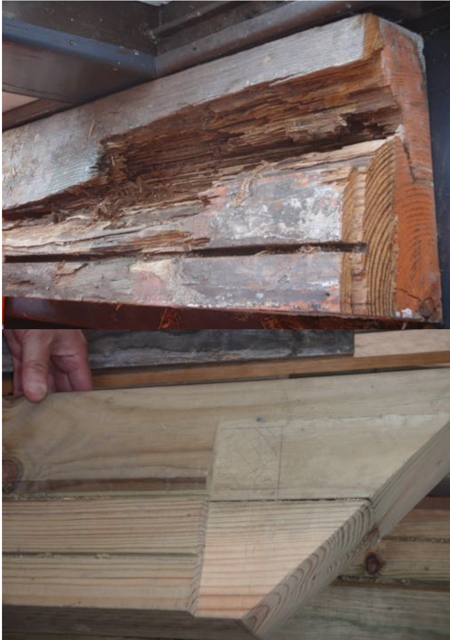
Figure A.101d: Rotten timber frame sections used as a pattern for fabrication of replacement timber frame sections, Princes Risborough North Signal Box. (Author 2018)
