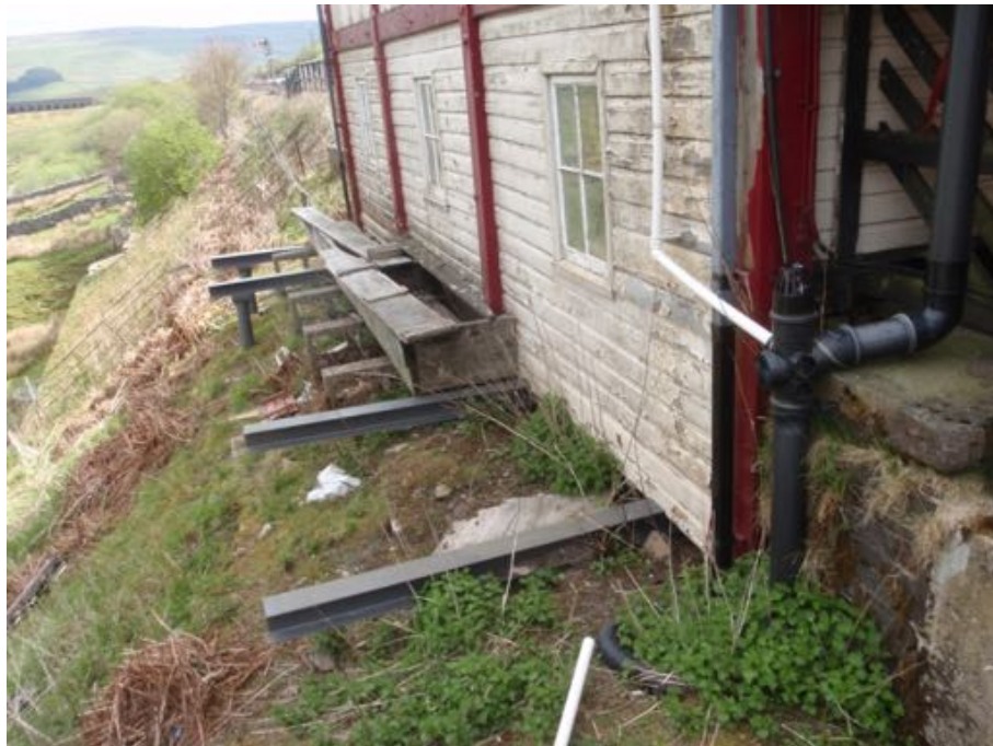
Figure A.51b: Piles and beams to prevent further structural movement of Garsdale Signal Box. (Author 2016)
