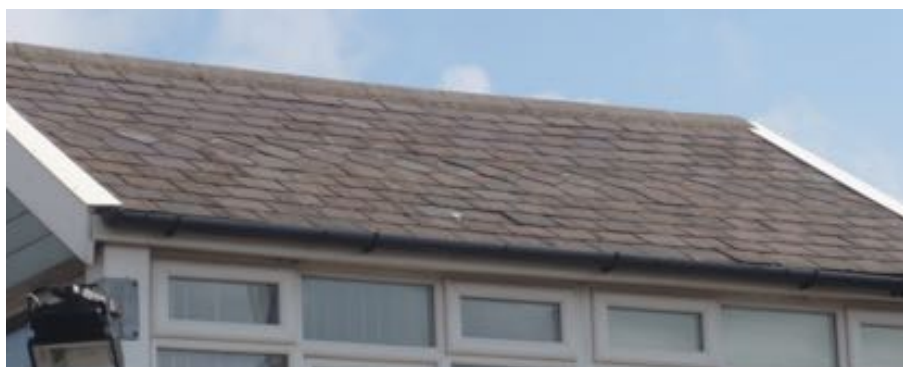
Figure A.92b: Roof detail for North Seaton Signal Box, retaining the diamond slate detailing redolent of original detailing despite the otherwise substantial evidential degrading. (Author 2019)
