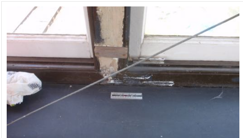
Figure A.101c: Movement prevention and monitoring using tension wire and tell-tale ruler with laser spot, Princes Risborough North Signal Box. (Author 2018)
