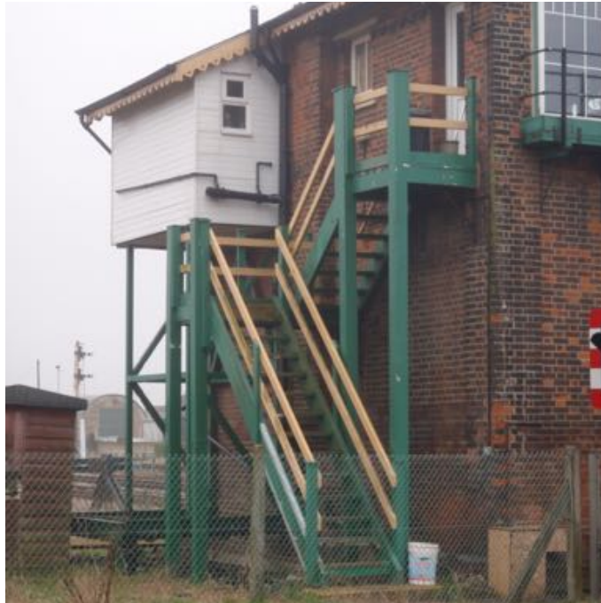
Figure A.81b: Rear elevation of March East Junction Signal Box, showing high-level toilet block extension and supporting structure. (Author 2018)
