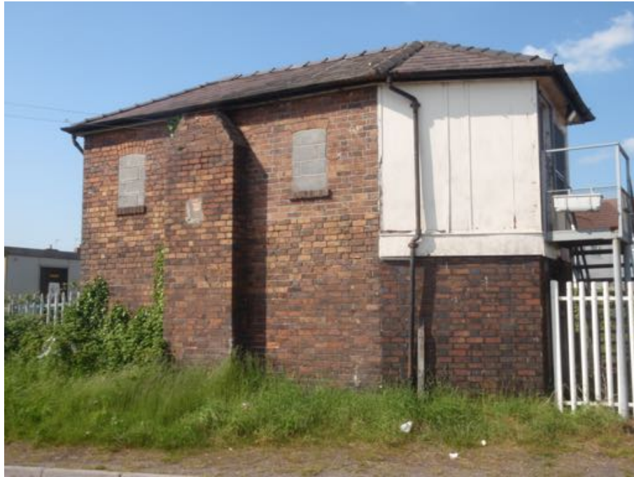
Figure A.75b: South elevation of Llanelli West Signal Box, showing chamfer at east end. (Author 2018)
