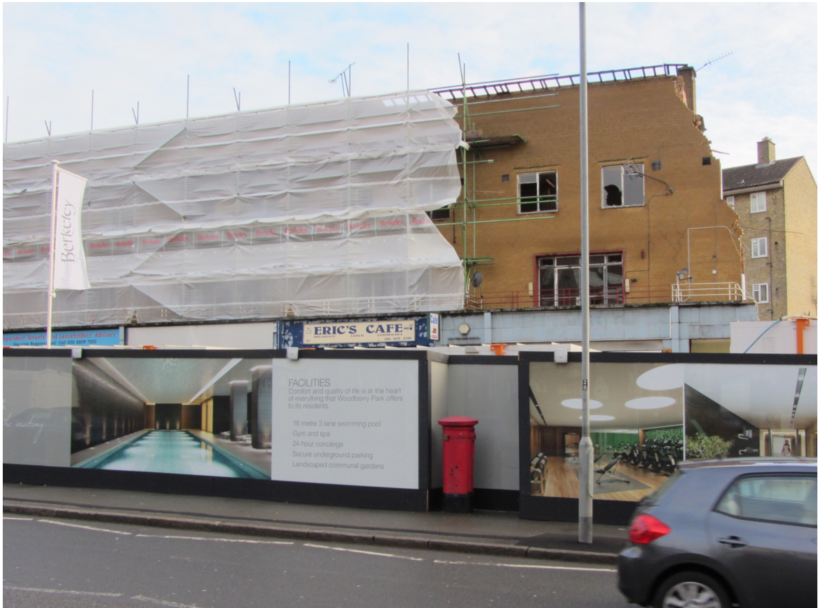
Figure 4: The parade of shops and homes above being demolished with hoarding advertising swimming pool for exclusive use of residents of a new private block
