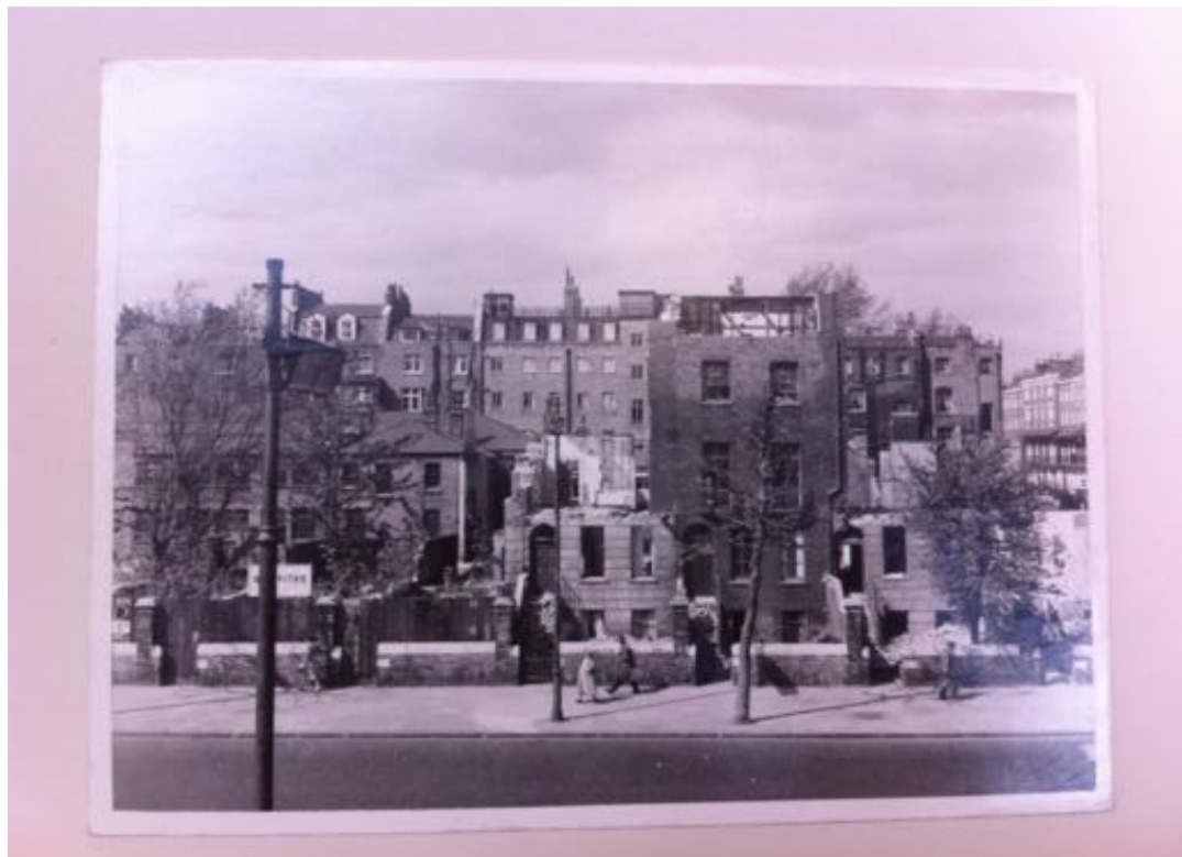
Fig. 6.6 Marylebone Road North side during demolition with the rear of Dorset Square beyond (SMS Archive/City of Westminster Archive)
