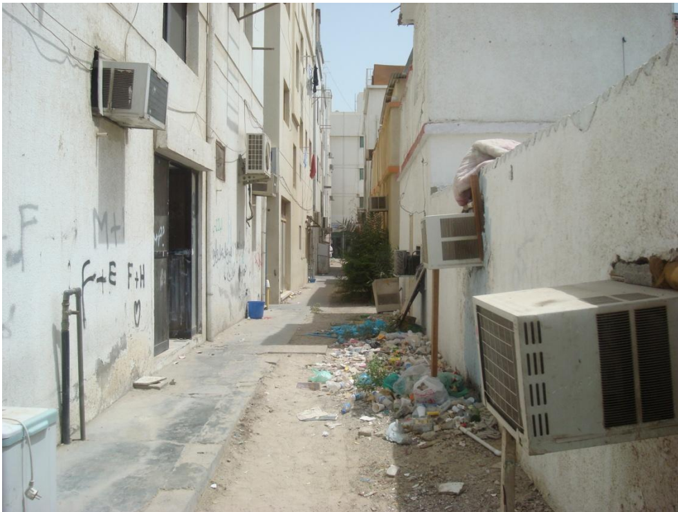
Figure B: An alleyway with dirt, graffiti, and a window unit that is about to fall
