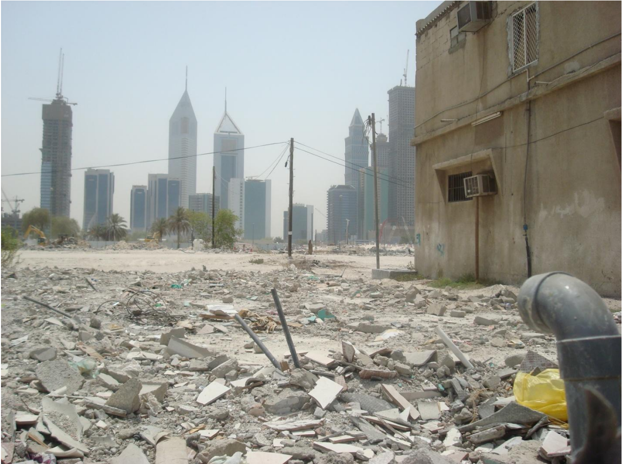
Figure A: In 2007, Al-Satwa was allocated to Meraas, a Dubai based real estate investment company, to generate a development comprised of hotels and skyscrapers. The firm started knocking down the area in 2008. Many workers moved to the surrounding areas like Al Jafiliya, Al Bada'a, and Al-Karama. People who possessed a property in the area were compensated. The company decided to turn the area into a luxurious development with skyscrapers and artificial water canals. But, due to the global economic decline, some officials stated that the project is deferred until further announcement. (Note: Photo Taken in August, 2008. All the previous pictures were taken in January 2008, and summer 2007 before demolition)
