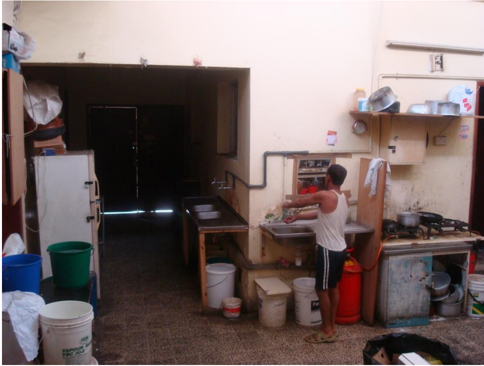
Figure A: A view from the porch towards the courtyard and main entrance. There are extensions of pipelines for multiple sinks to serve large numbers of occupants.
