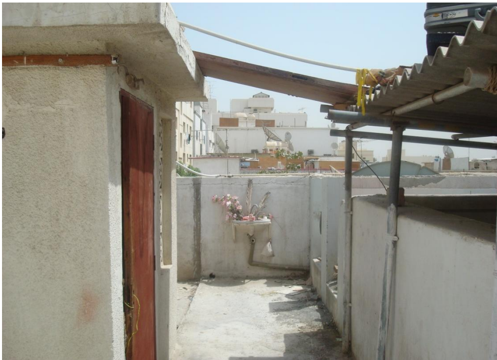
Figure B: To the left, a door that leads to the staircase; to the right, asbestos panels covering the courtyard.
