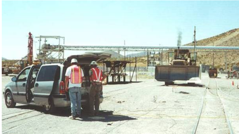
Figure 2.8 A bulldozer Used as a Seismic Source to Perform SASW Test at Waste Handling Building (WHB) at Yucca Mountain, NV
