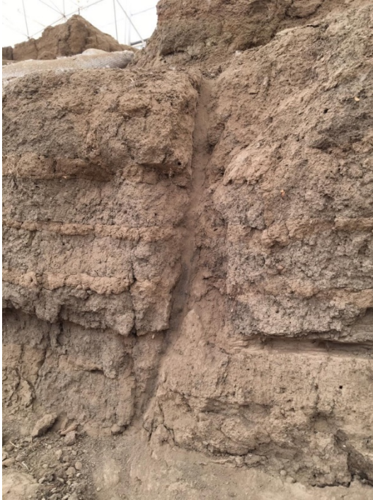
Figure 31: Wall repair in Building 132, central crack filled with perlite, 10% Paraloid B-44 w/v in 50:50 acetone ethanol mixed with sieved soil.
