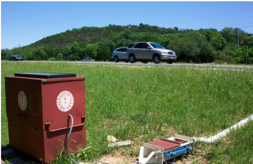
Figure 39: Photograph of H-flume and drainage pipe at Loop 360 monitoring site
