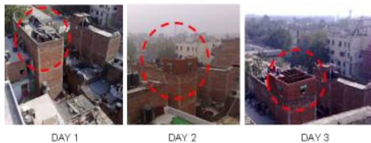
Figure 6. Overnight rampant constructions and additions to existing buildings
