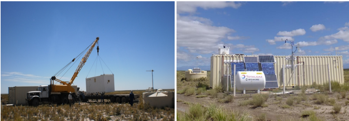
Figure 2: (Left) Replacing the old CLF container. (Right) The CLF after the upgrade was completed.
