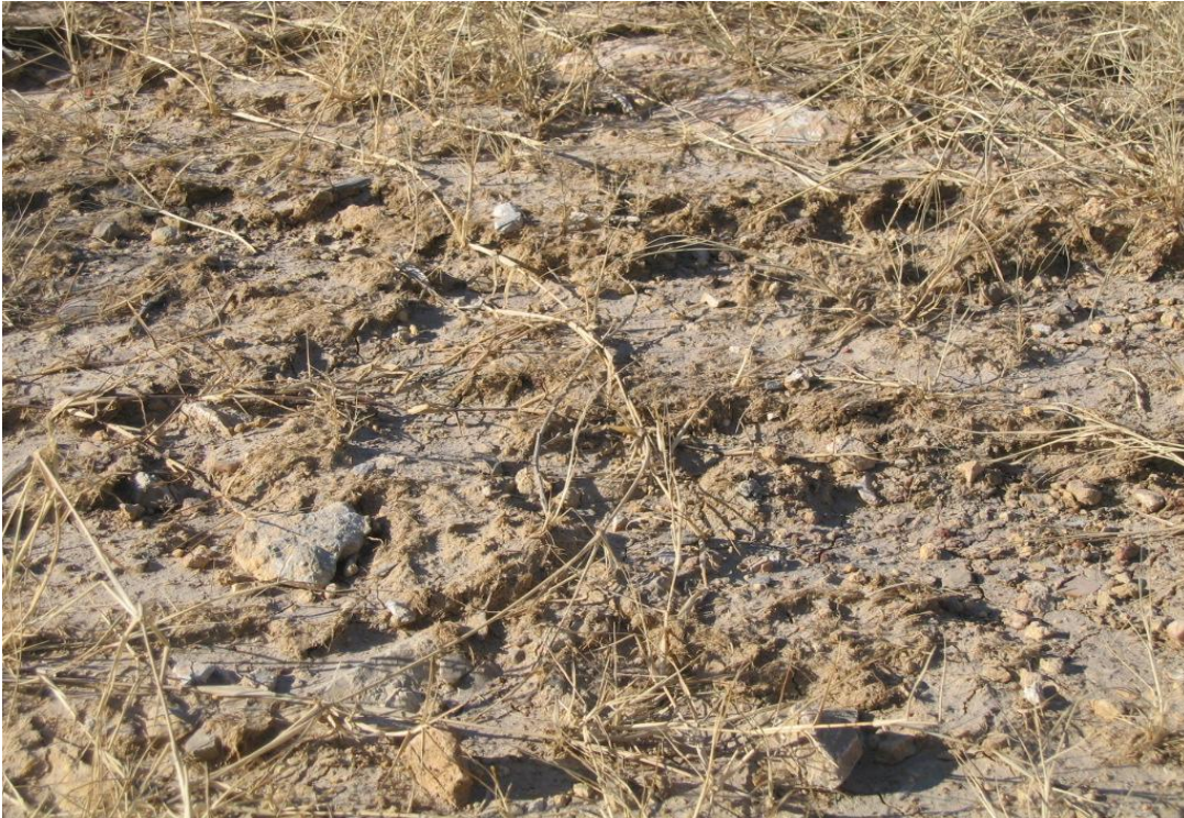
Close-up View of Scouring Occurring near the Bottom of VP07
