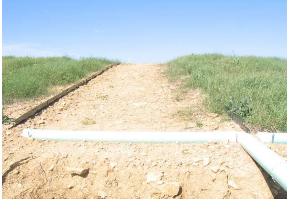
Figure 4-3 Example of vegetation encroachment
