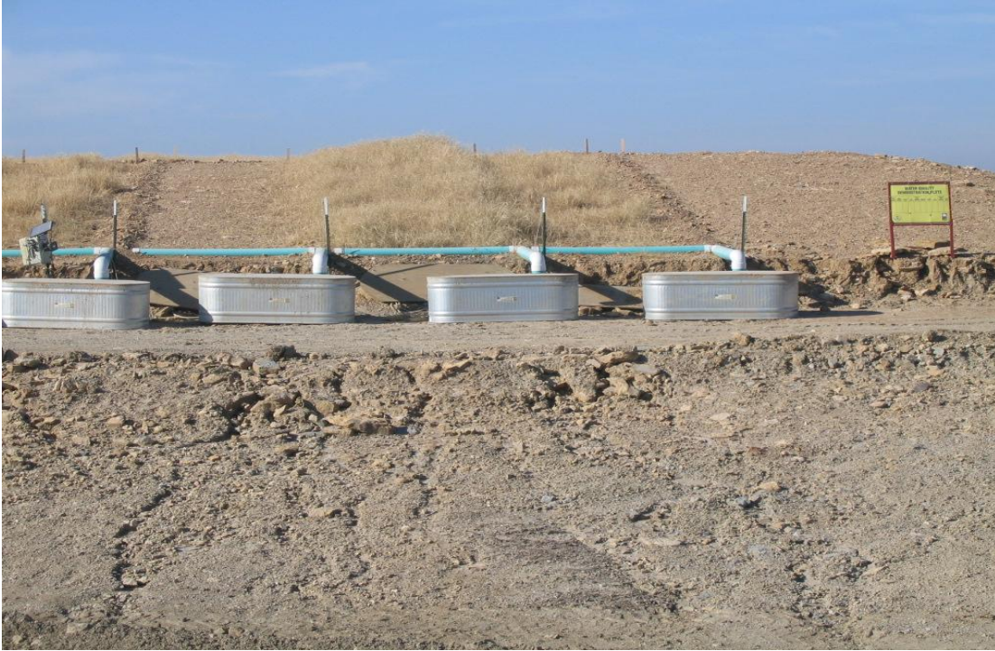
Figure A-73. Composite view of test plots VP07 (partial view), VP08, VP09, and VP10 taken December 14, 2006.
