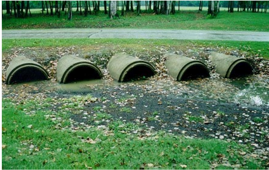
Figure 3.6: Blocked culverts in the upstream part of Addicks Reservoir
