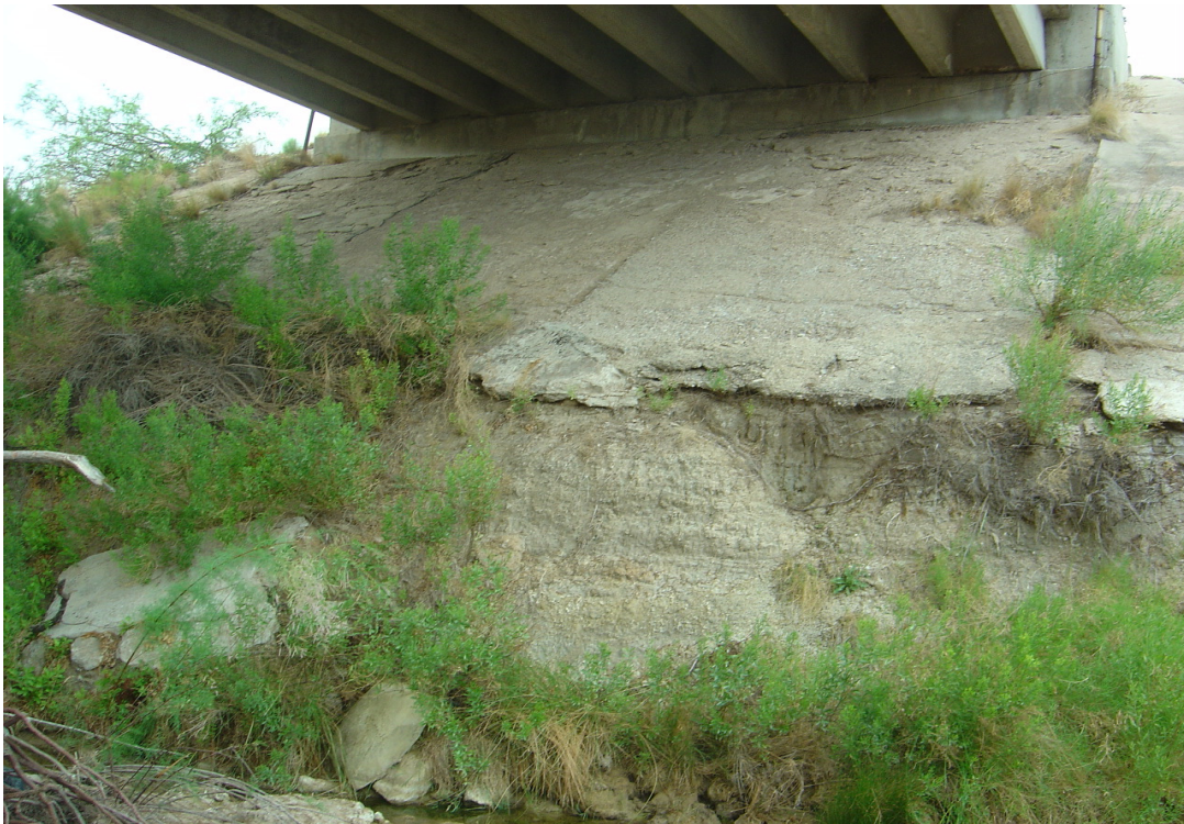
Figure 5-10: Deteriorated riprap at Site 32 located on FM 652 in the El Paso District
