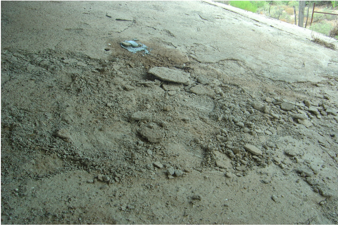
Figure 5-9: Riprap deterioration at Site 31 in the El Paso District
