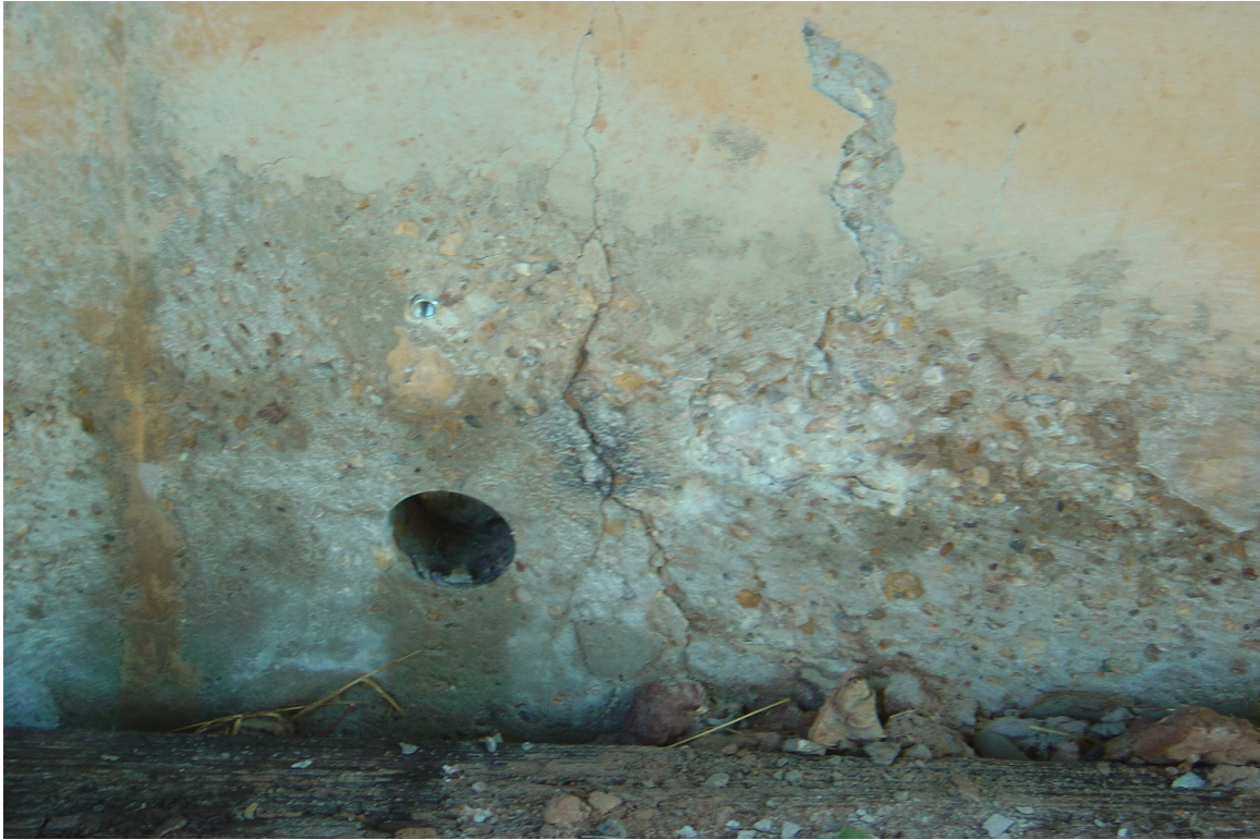
Figure 5-3: Damage to the lower part of a wall below US 83 in Childress District
