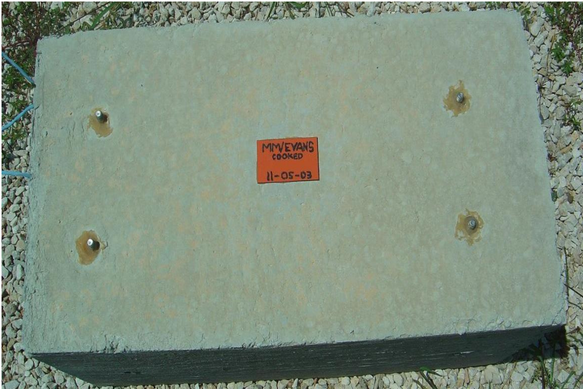
Figure 2-1: Exposure block containing non-reactive aggregates and heat cured up to 183 °F (83 °C), showing no signs of distress after 3 years
