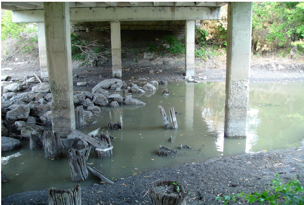
Figure 5-7: Deteriorated concrete columns from a bridge in the Paris District
