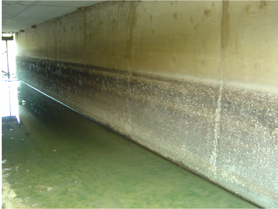
Figure 5-5: Deterioration commonly found in culverts in the Paris District. The distress begins near the base of the culvert and continues up the side, likely in line with the highest level of water.
