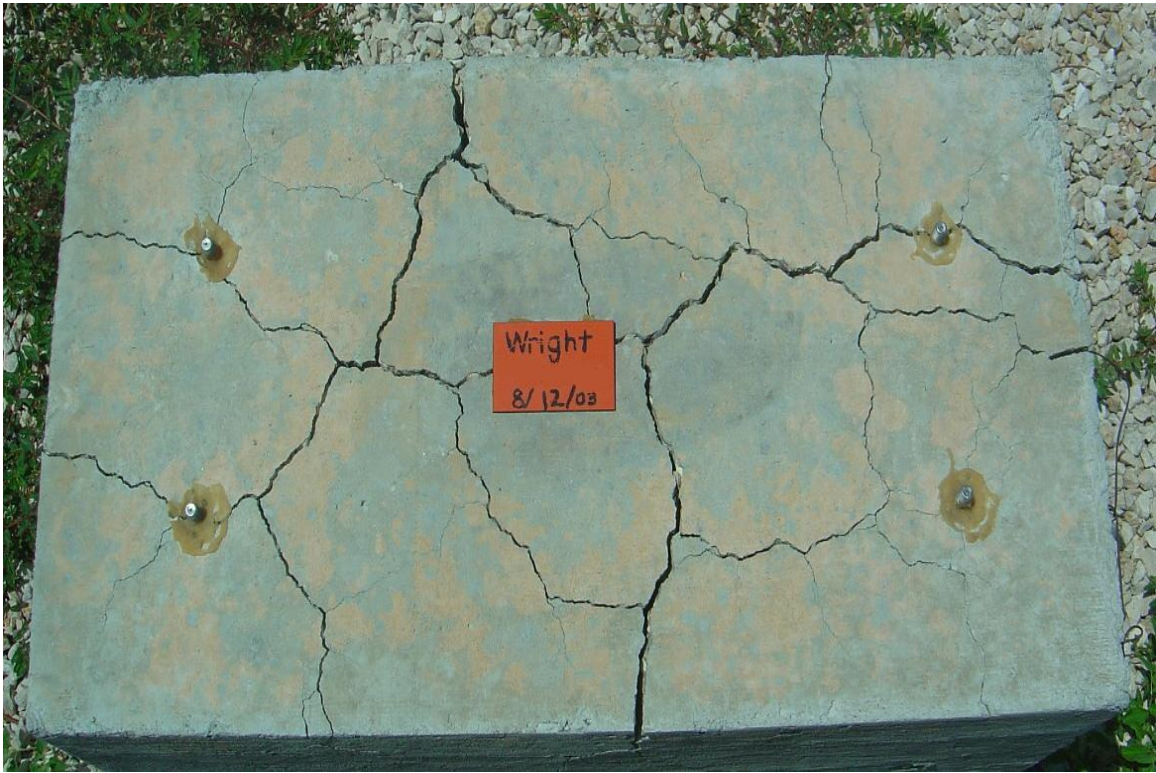
Figure 2-2: Exposure block containing highly-reactive aggregate and heat-cured up to 183 °F (83 °C), showing signs of significant cracking after 3 years
