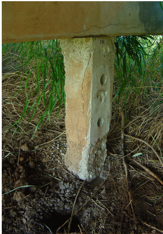
Figure 5-4: Damage to a bridge column on FM 2278, south of Childress, Texas
