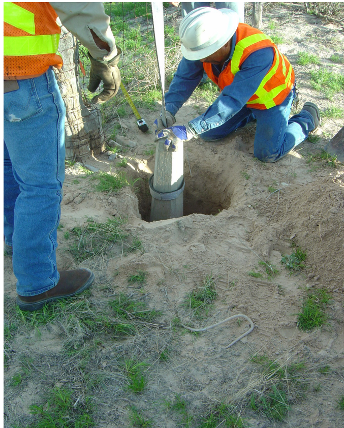
Figure 5-13: Placement of new ROW marker in the existing location of the deteriorated ROW marker
