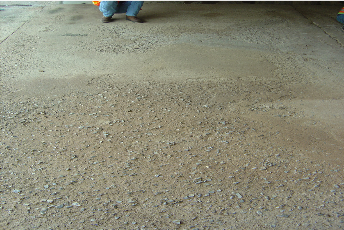
Figure 5-8: Riprap deterioration occurring on the embankment below a bridge
