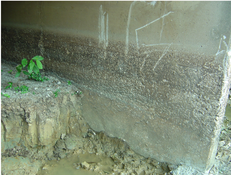
Figure 5-6: Deterioration of a culvert above the soil level, with no deterioration visible below the level of the soil (after excavation).
