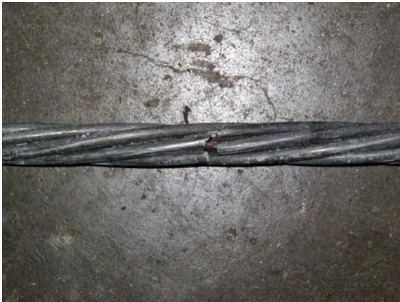
(c) Wire fracture at the midspan
