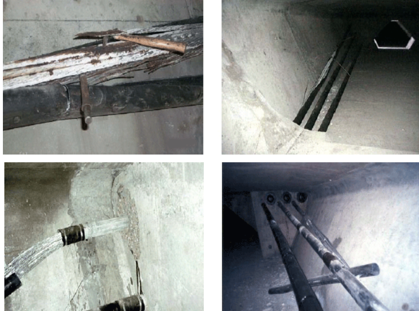
Figure 1.3 Corrosion Damage Observed on the Mid-Bay Bridge (FDOT 2001)
