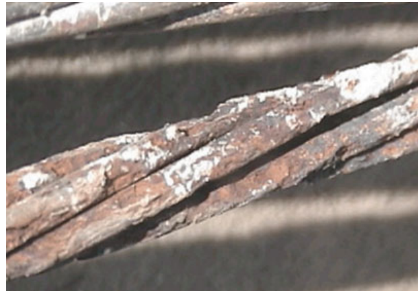
(b) Severe Pitting
