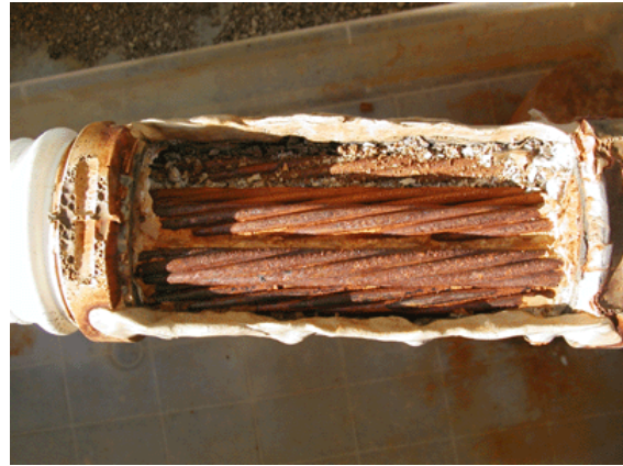
(f) Corrosion products after rain evaporated
