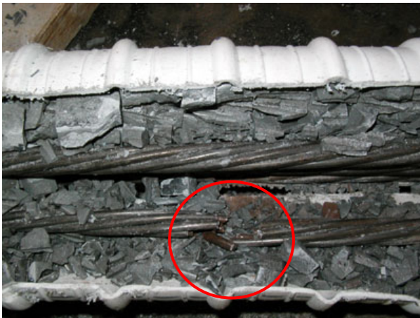
(a) Condition of grout near fractured wires
