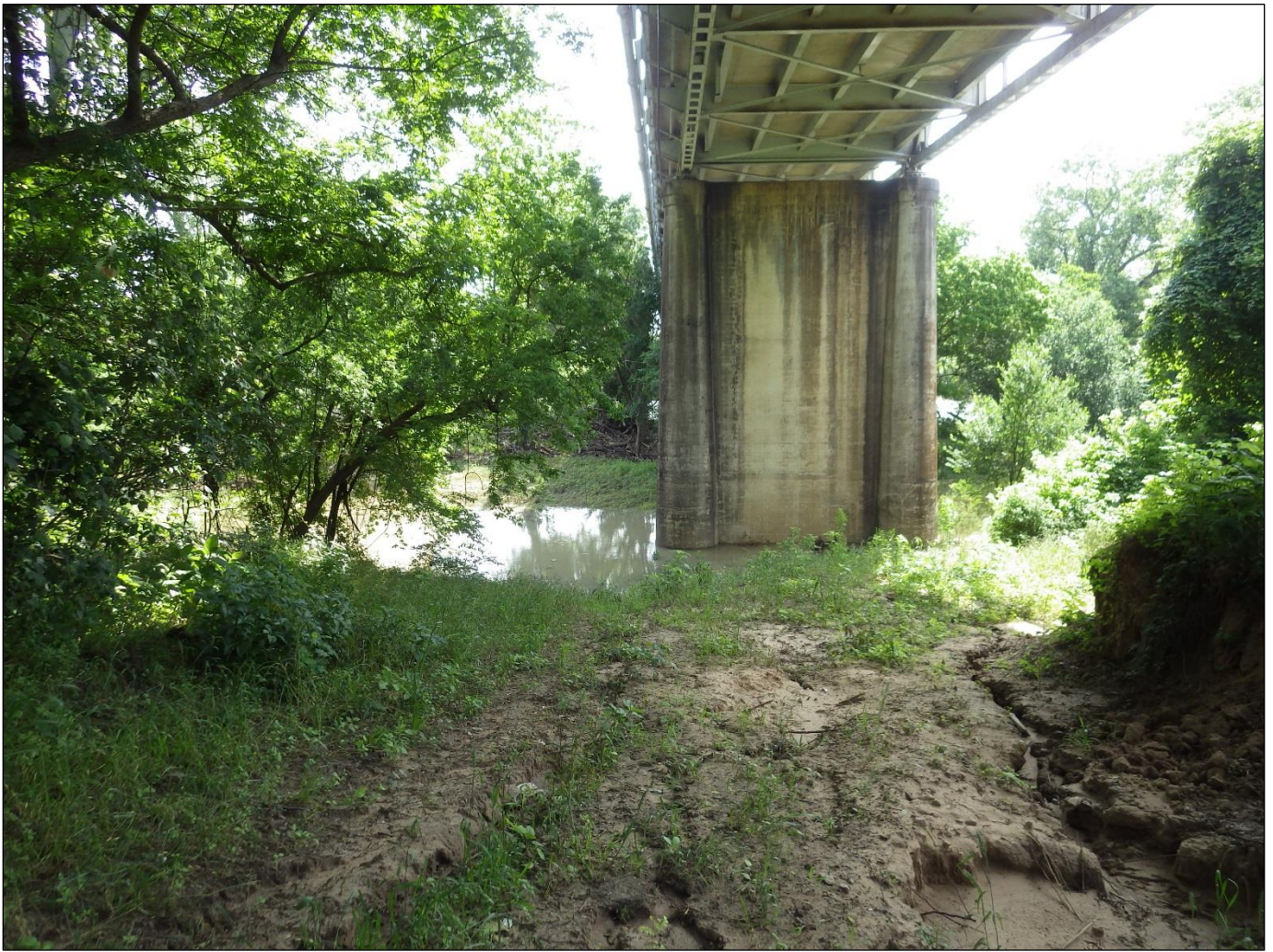
Figure 23. Eroded area beneath the BS71E bridge within the northwest quadrant. Note high water from recent flooding.
