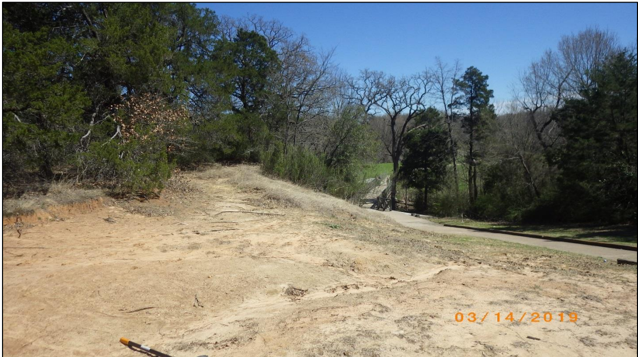
Figure 14. Erosion to subsoil on the first terrace of the west bank of Prairie Creek. View is to the east.
