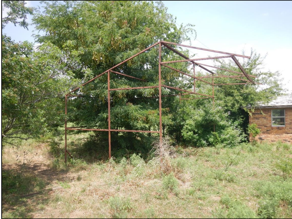
Figure 19. View of the metal frame adjacent to the brick outbuilding; view northeast.
