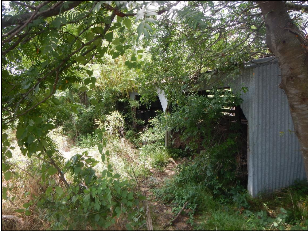
Figure 27. View of the southern end of the barn showing the overhang; view southwest.
