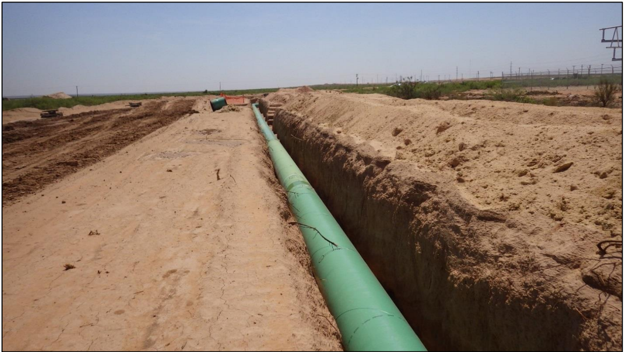
Figure 13. Pipeline installation at the southern end of the Riverton Sw. – Tunstill POD route, photo taken facing east.
