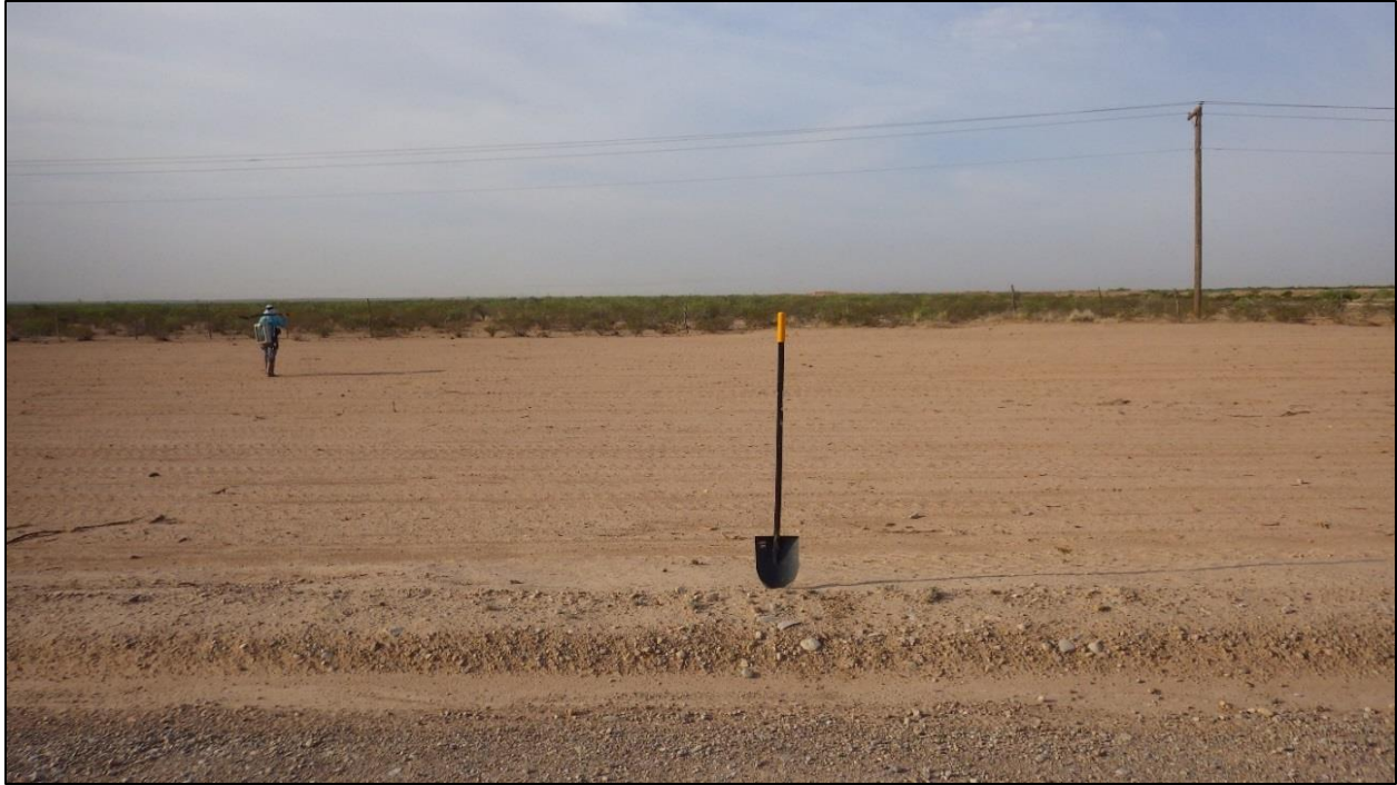
Figure 8. Pipeline installation that crosses into the Riverton Sw. – Tunstill POD ROW south of SH652, photo taken facing south.
