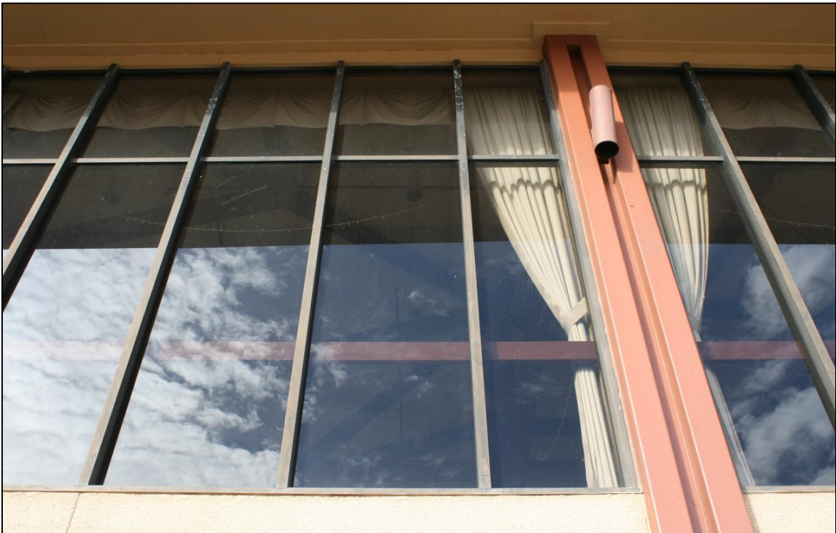
Figure 11. Detail of the upper level windows and steel pilasters of the center wing.
