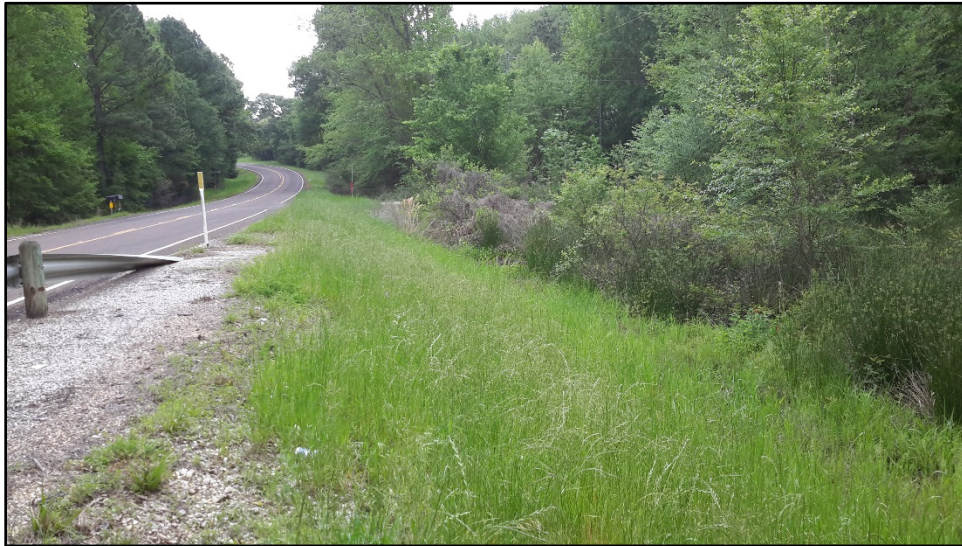
Figure 8. South side of FM 1511, on the east bank of Resaca Creek facing southeast. Note the steep raised road grade with standing water wetlands at base (right), utilities are marked along this side, but are not visible in this picture.
