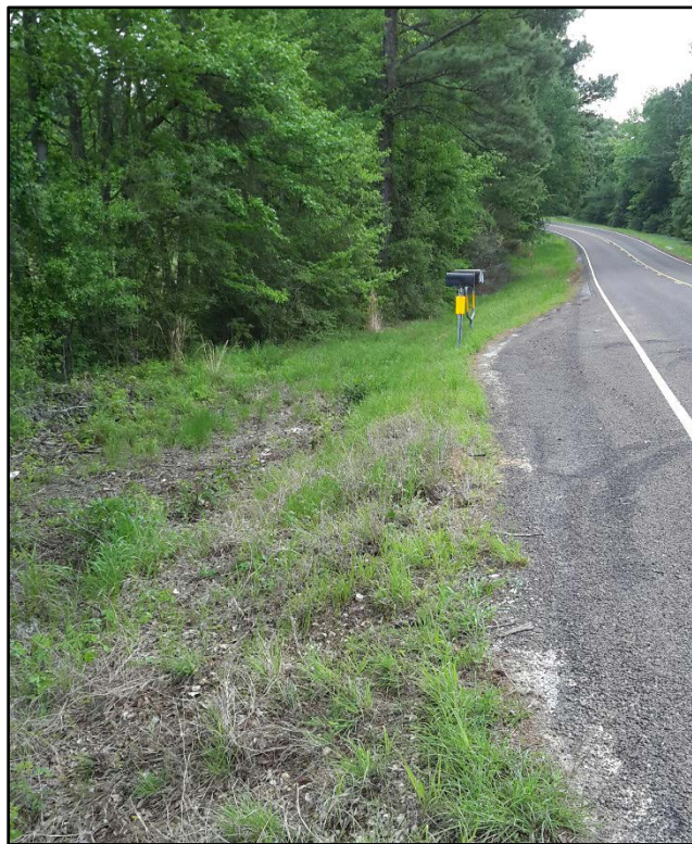
Figure 9. North side of FM 1511, on the east bank of Resaca Creek facing southeast. Note the steep raised road grade. The saturated ground and wetland grasses (right) are located near a standing waterbody (just left of view) from a culvert just east of the bridge.
