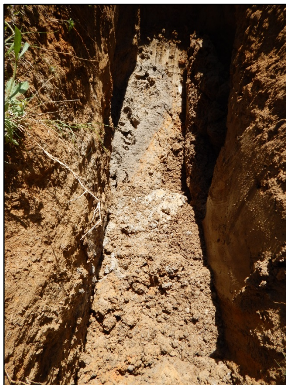
Figure 11. BHT1 trench floor with wall collapse and water table filling the trench, facing northwest.
