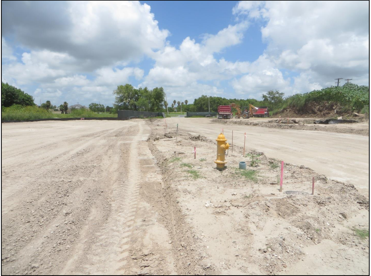
Figure 1-6. View of a utility line that runs along the southern edge of the new road.
