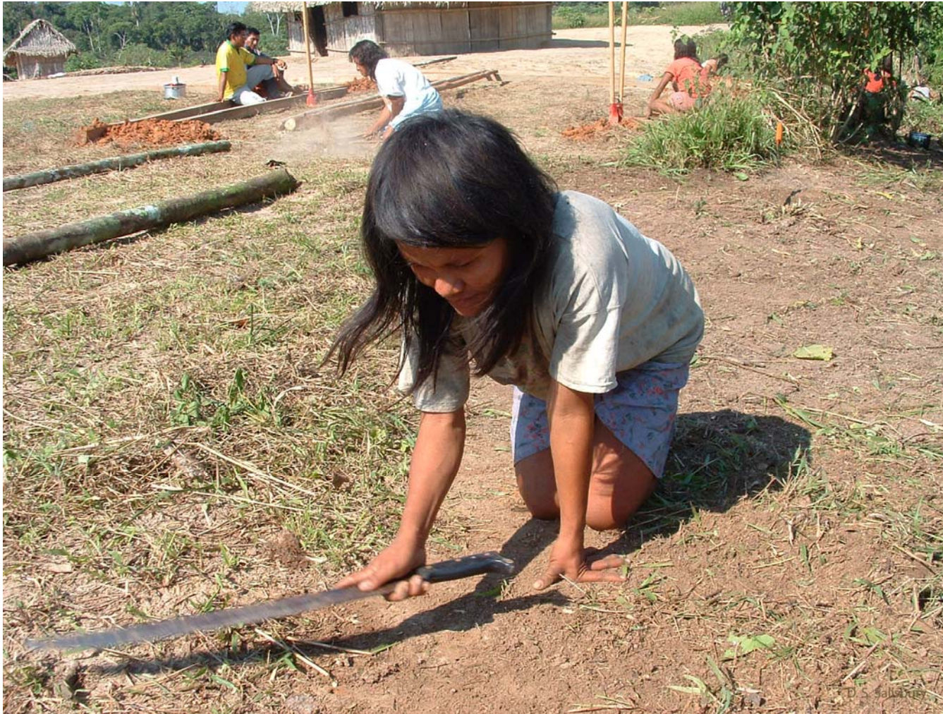
Figure 83. Women contribute as well to the construction of the new house. Here Tamila clears the vegetation in the future yard of the house. In the background other women and children work.
