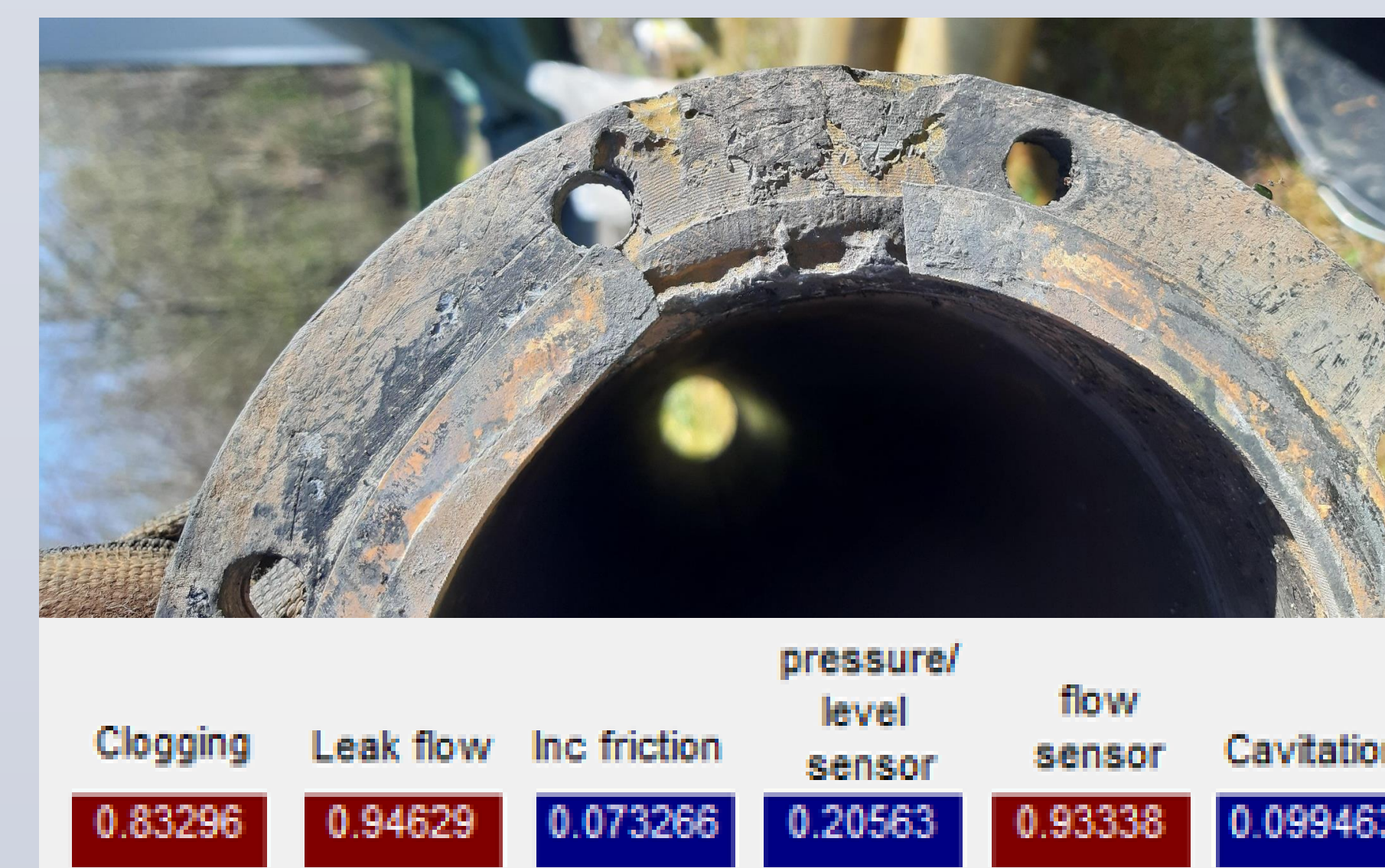
Fig 3: Leak in the riser. The fault leads to decision variables "clogging", "leak flow," and "flow sensor fault" close to 1.
