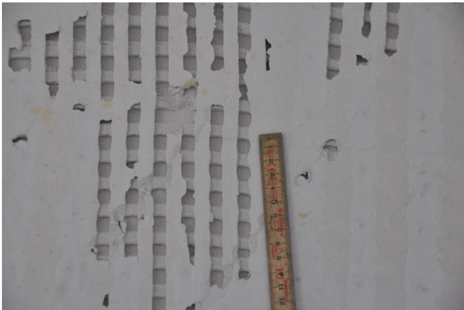
figure 14: Close up of the wall in figure 13 showing the size of the areas with no bonding. According to the producer, opening of max 4x4 cm are accepted © AAU
