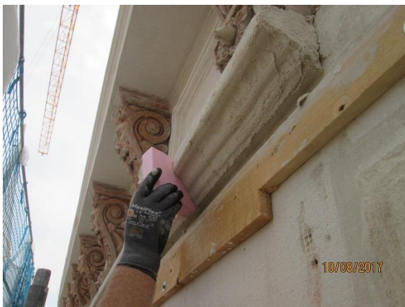
figure 130: Impressions from the work on the aerosol insulated façade, © Trimmel Wall Architekten ZTGmbH
