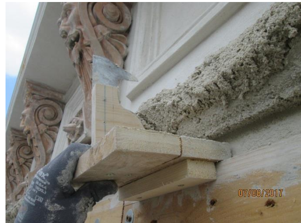
figure 129: Impressions from the work on the aerosol insulated façade, © Trimmel Wall Architekten ZTGmbH
