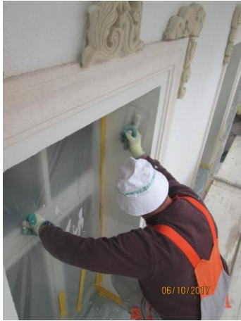
figure 132: Impressions from the work on the aerosol insulated façade, © Trimmel Wall Architekten ZTGmbH
