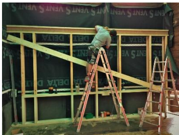
figure 66: Black wind paper and frame construction for the OSB panels © DI Hans Peter Gruber
