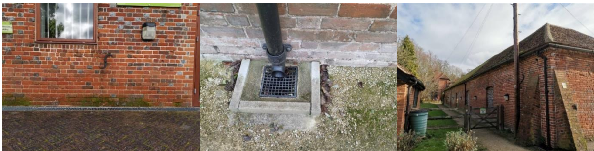
figure 93: Channel drain © Athina Petsou figure 94: Detail of drainage system © Athina Petsou figure 95: Gutters and downpipe on north façade © Athina Petsou
