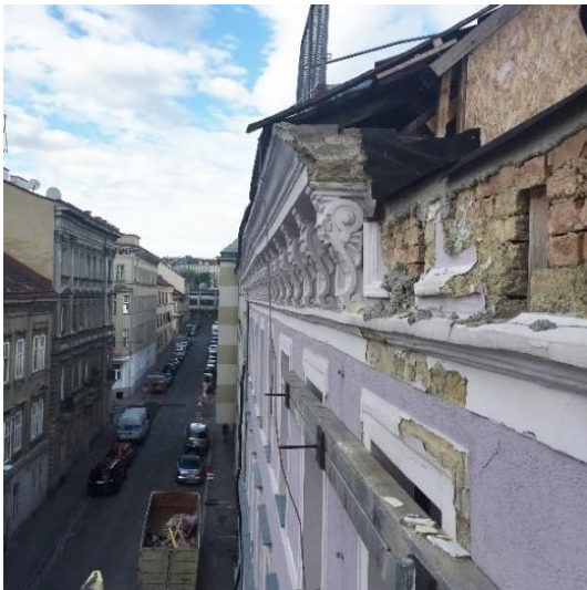
figure 124: Damaged façade, © Trimmel Wall Architekten ZTGmbH
