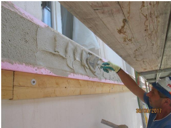
figure 128: Impressions from the work on the aerosol insulated façade, © Trimmel Wall Architekten ZTGmbH
