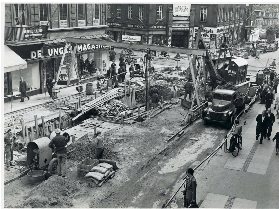
Fig. 2. District heating construction works, Aarhus. Picture source: Affaldvarme Aarhus. Reprinted with permission.
