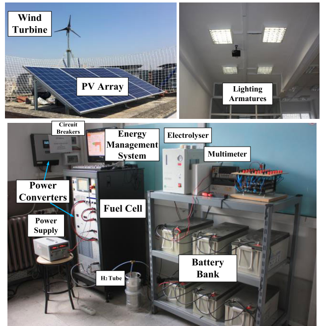
FIGURE 16. Experimental setup of laboratory scale microgrid system.
