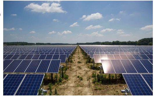
Figure 1: Solar farm in Louisa County (Photo credit: Dominion Energy)
