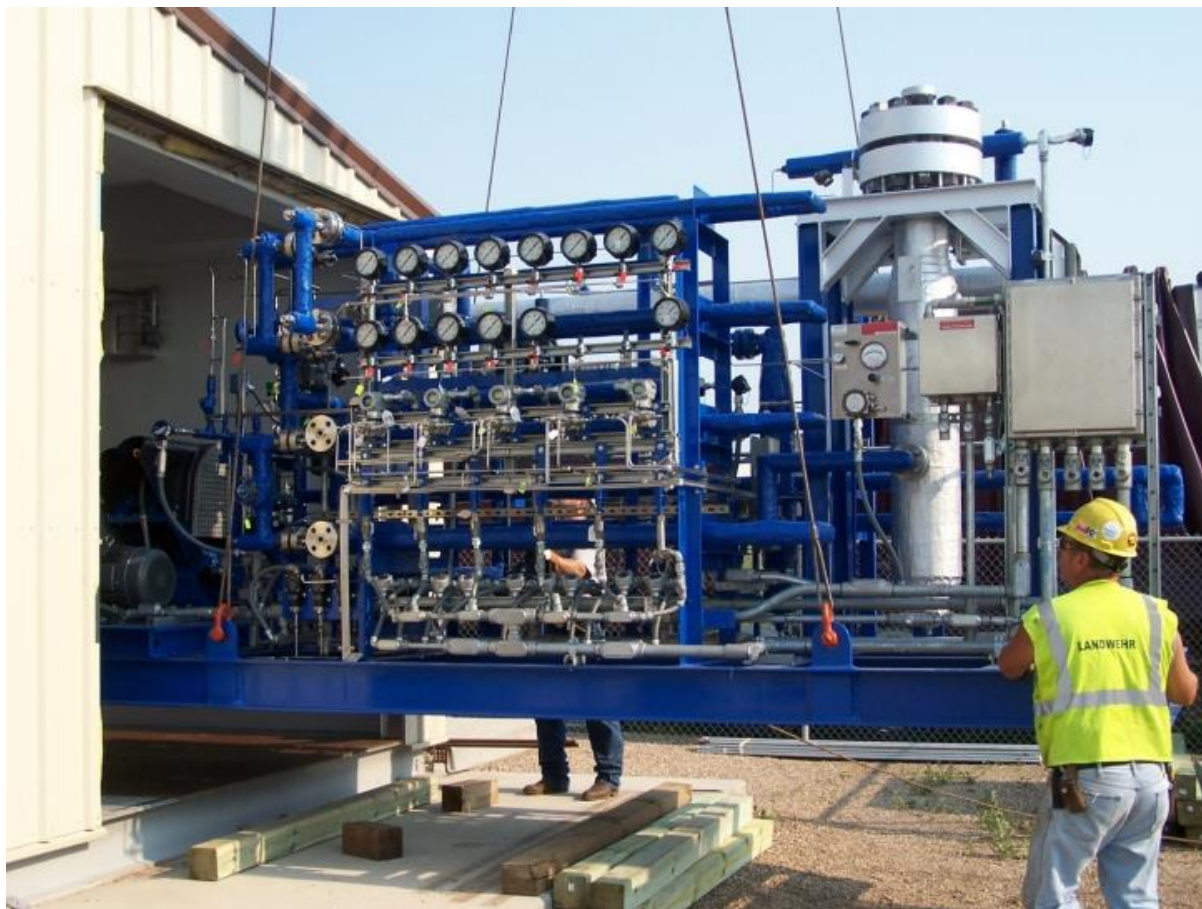
Figure 29. University on Minnesota Ammonia Reactor Skid
