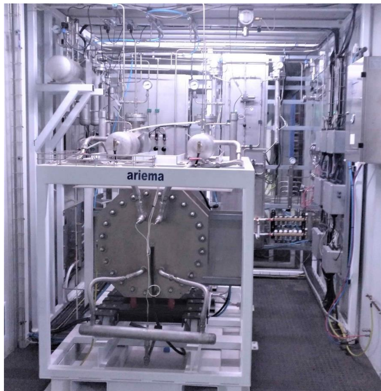
Figure 33. Ariema PEM Electrolyzer
