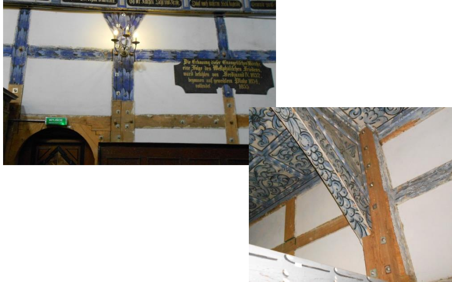
Fig. 12 Timber-to-timer interventions in a church in Jawor, Poland built with traditional timber frames (credits: E. Poletti).
