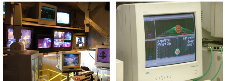
Figure 4. Primary breakdown of logs: headrig control room. (Courtesy of Weyerhaeuser Inc.)
