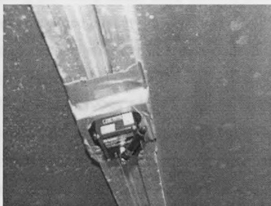
e) Triaxial Accelerometer Trailer Ceiling
