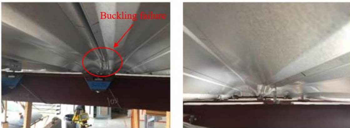
Figure 2.15: Deformation of panels subjected to uplift wind loads (Nasiri, 2019).
