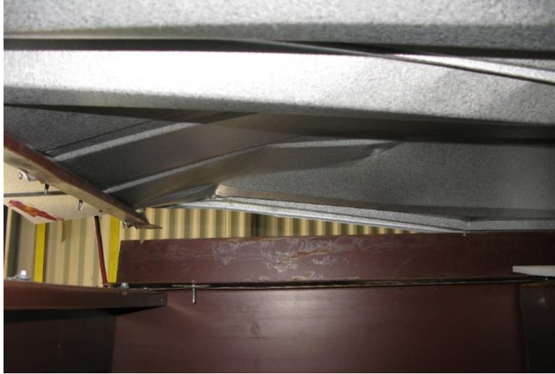
Figure 4.15: Edge failure as the SSMR was subjected to pressure.
