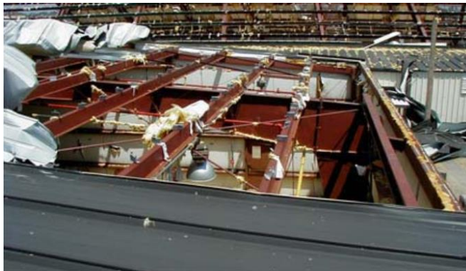
Figure 1.4: Roof failure during extreme wind events (Dixon and Prevatt, 2010).
