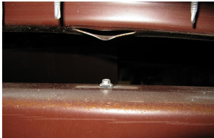
Figure 4.22: Fastener failure at the eave edge (experiment 3).
