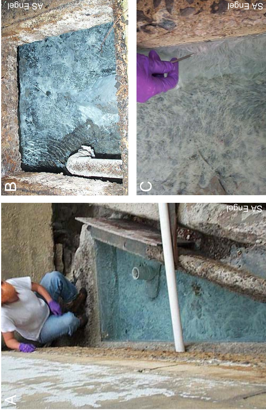
Figure B-4: (A) Microbial mats coating a concrete discharge pool from the Sulphur Temple bathhouse, White Sulphur Springs, Sharon Springs, Schoharie Co., New York. (B) The pipes running from the bathhouse were exposed under access panels. (C) Long filaments on concrete.
