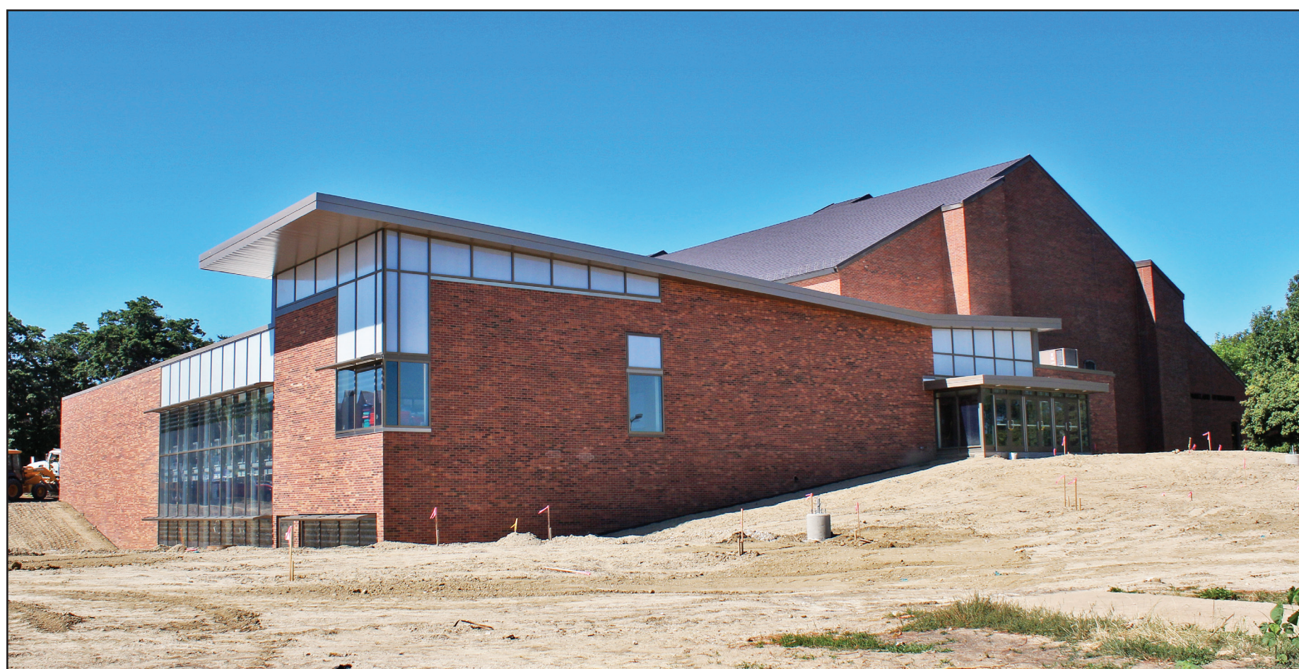
Construction continues on the Parkland Fitness Center addition June 22, 2012. The facility is now open for use, although finishing touches are still being completed on the exterior.
