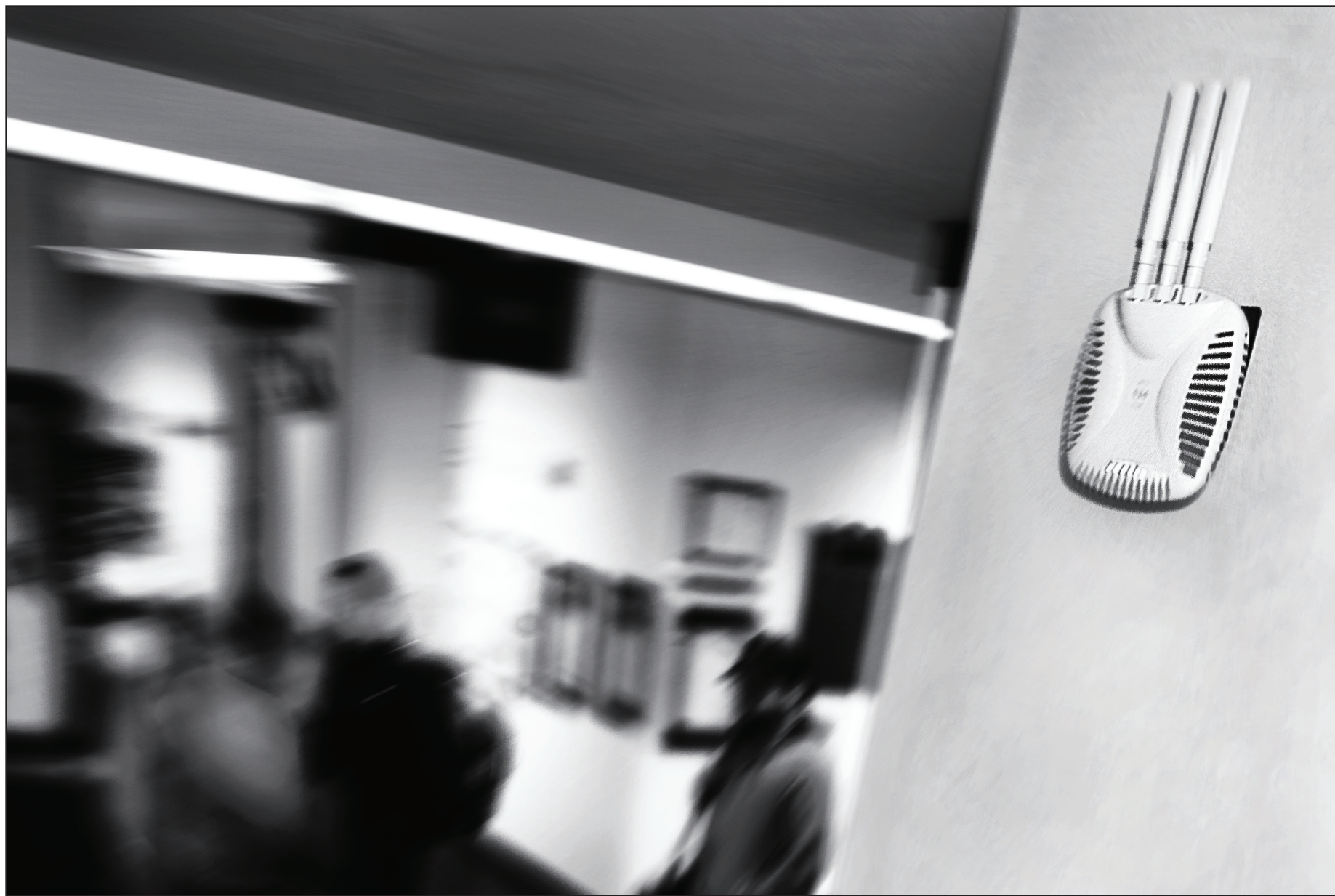
Photo Illustration by Briana Kay Stodden/Prospectus News Parkland College has replaced Wi-Fi access points and added new devices all across campus. The installation will increase the overall coverage area and the saturation capability of the wireless internet network.
