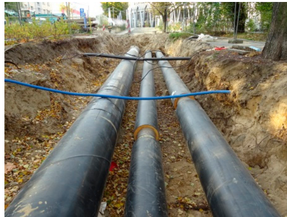
Figure 1. Example of pre-insulated heating pipes located in the ground layer at a depth of up to 1 m.
