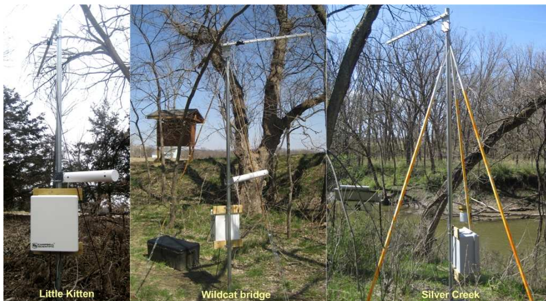
Figure 5.27 Gateway stations at Ft. Riley site, KS
