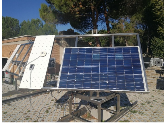
Fig. 3. Outdoor IRT testing bench at the Photovoltaic Solar Energy Unit of the CIEMAT, in Madrid.
