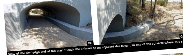
View of the dry ledge and of the way it leads the animals to an adjacent dry terrain, in one of the culverts where this solution was implemented.
