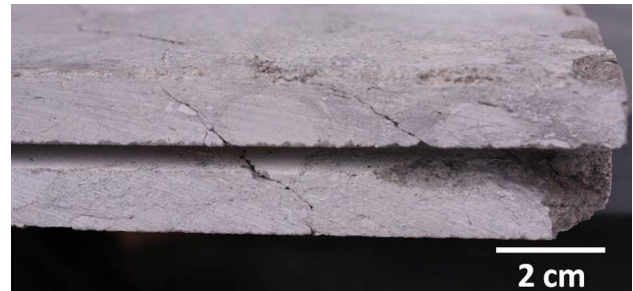
Fig. 4 Fractures and loss of material on AV slab in the kerf/slot region where the slab interacts with the anchoring system
