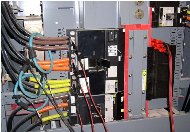
Figure A.3: 1200 Amps Molded Case Circuit Breaker Power Loss Measurement
