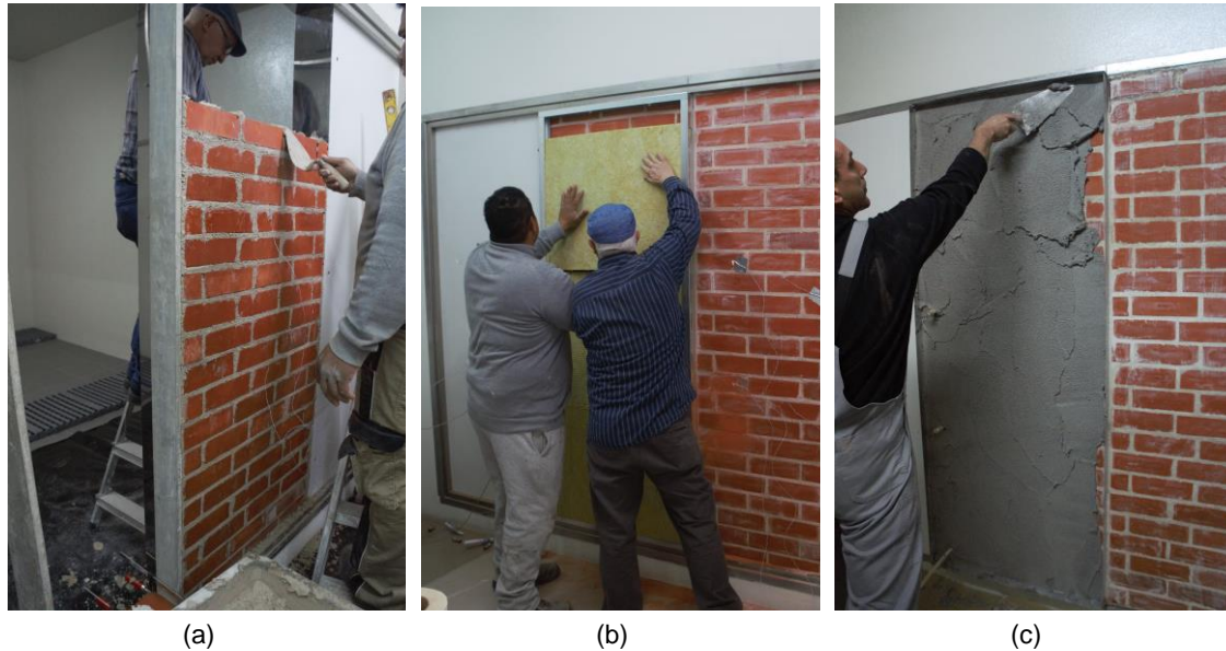
Figure 35. Construction of wall test specimens: a) construction of the solid brick masonry; b) application of the mineral wool on the interior surface of wall A; c) application of the insulating render on the exterior surface of wall B.
