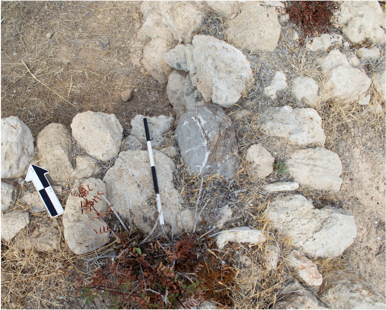
Fig. 5. Wall A in Room 2 of the Courtyard Building does not bond with the other exterior walls.
